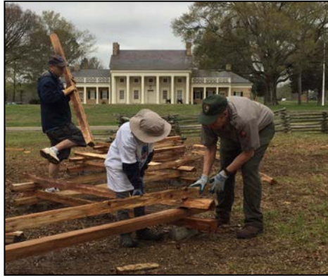
Volunteers assist Jim Szykowski, the park's chief of resource management, as they lay new fence rails on the historic McDonald Farm. NPS Photo
