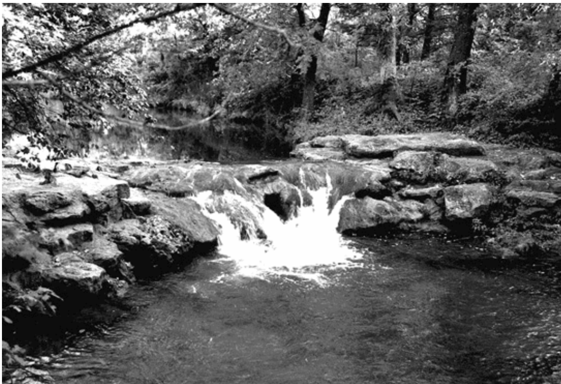
Central Campground Dam, looking east or upstream, circa 1999. (CNRA archives, LCS photo).
