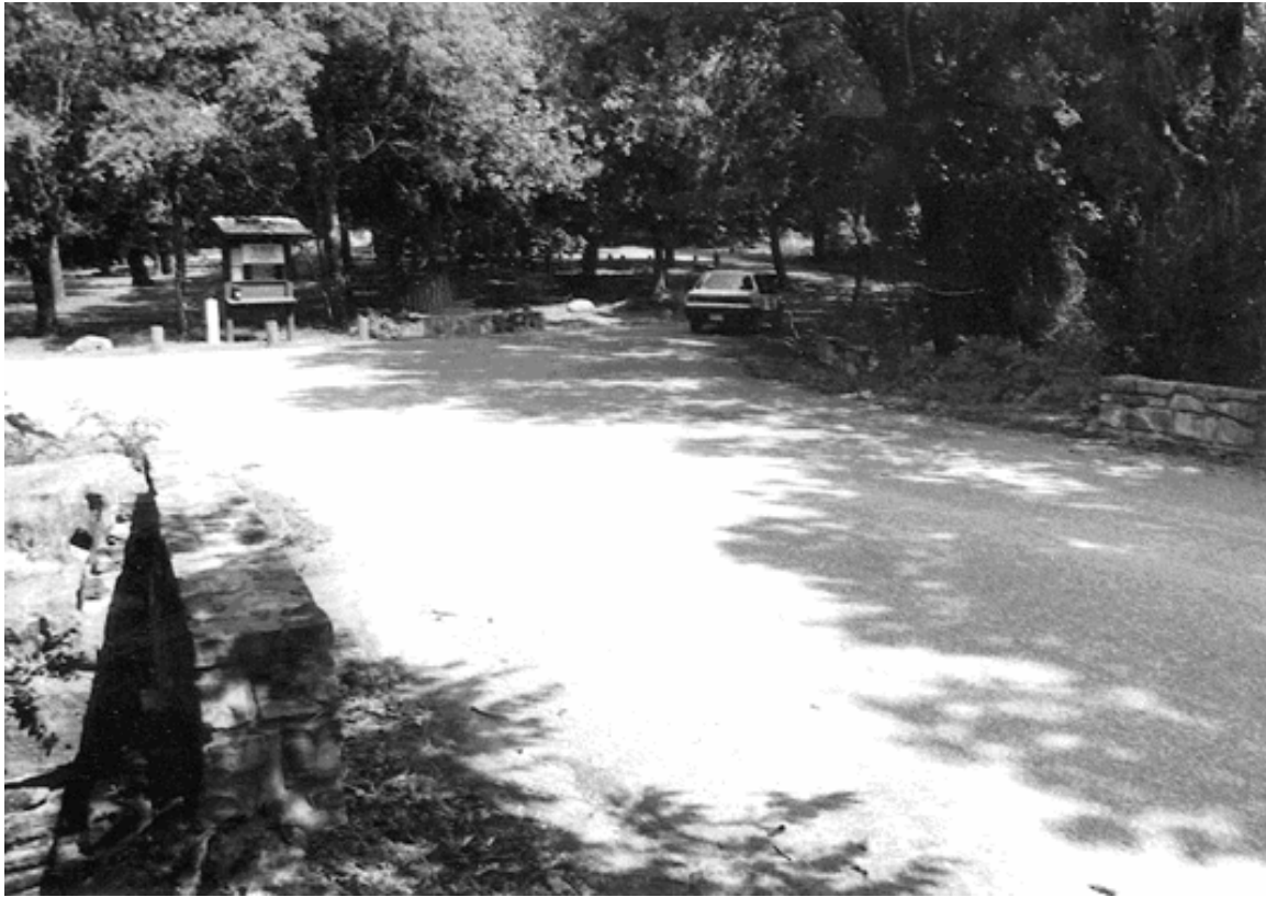
(Central Campground box culvert at entrance to southeast loop, circa 1995. (CNRA archives, LCS photograph)
