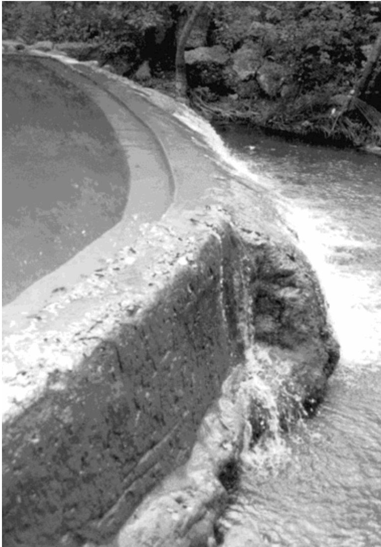
Detail of Concrete dam with travertine accretion (now lost) Panther Falls, circa 1999. (CNRA archives, LCS photo).
