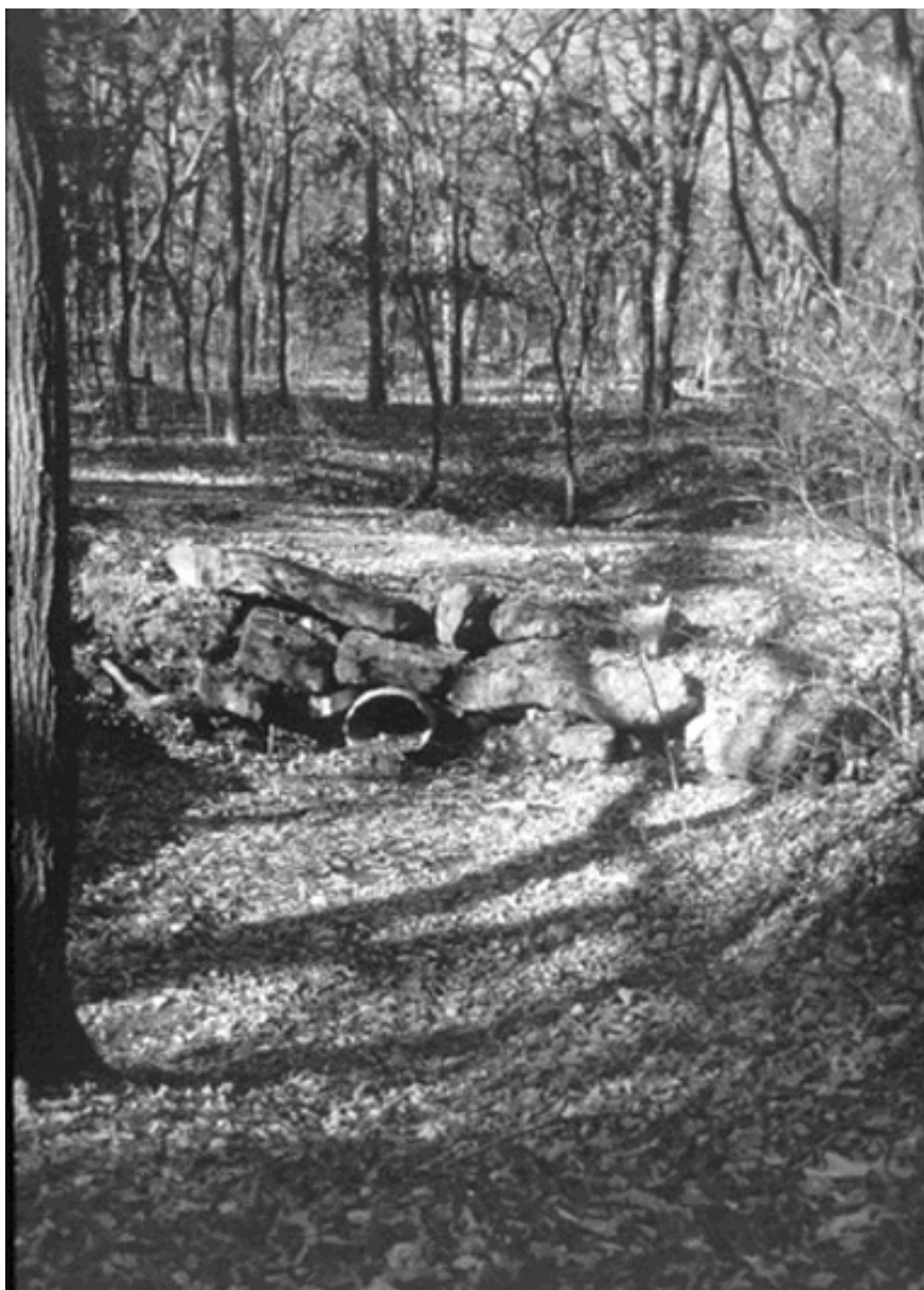
Dry-laid drainage culvert headwall, located along loop road, 2000. (Photography by Harlen Groe)
