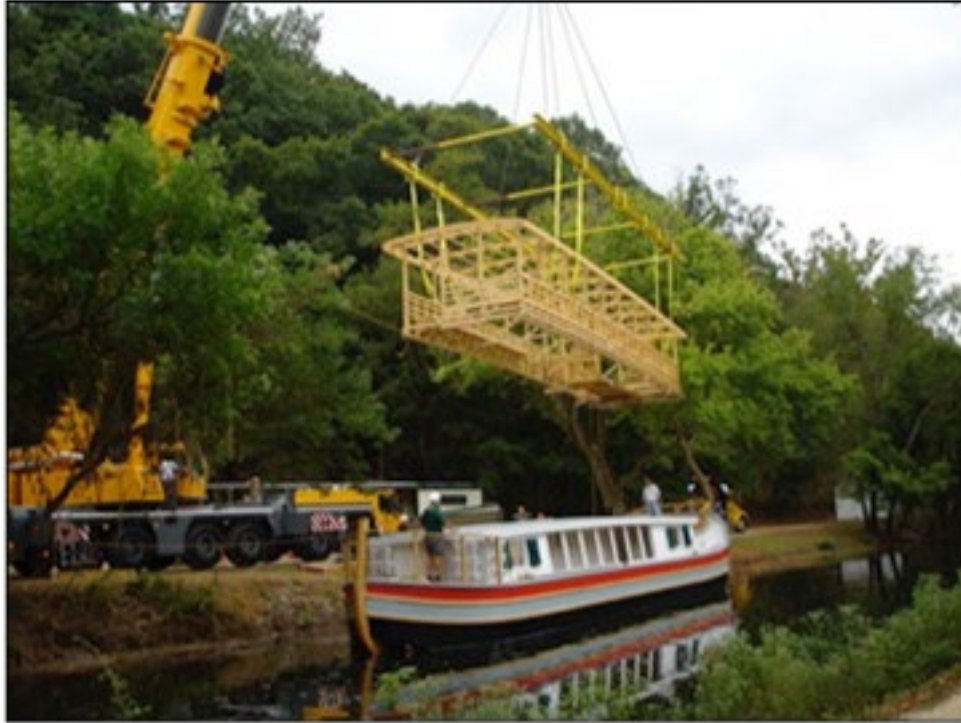
FIGURE 3.1: View of Charles F. Mercer Replica Canal Boat During Construction (Friends of the Historic Great Falls Tavern, 2015-2018)
