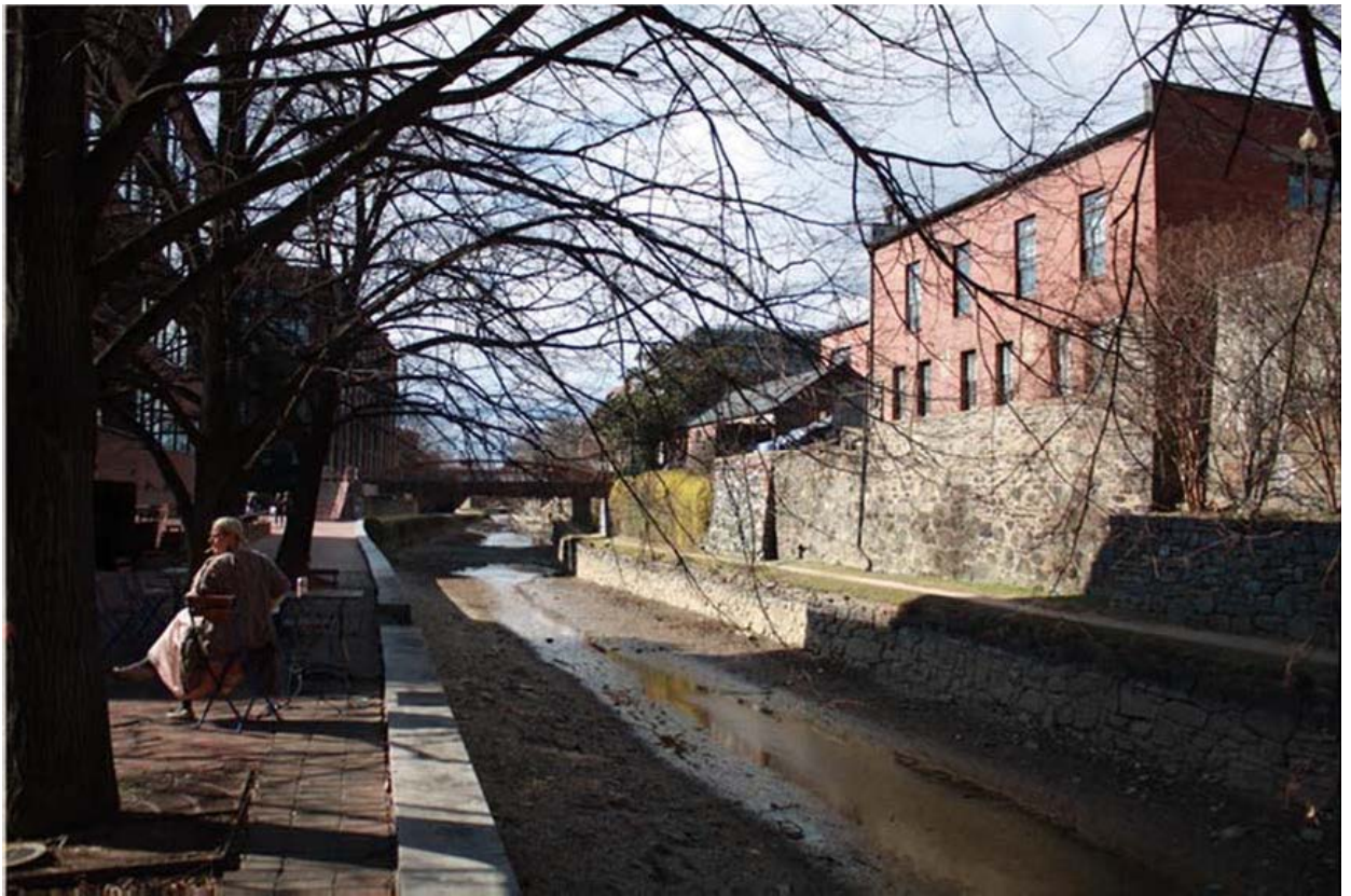
River side of the canal looking west at Fish Market Square. The historic retaining wall composed of stack stone with mortar is on the right side of the image (NCR CLP 2017).
