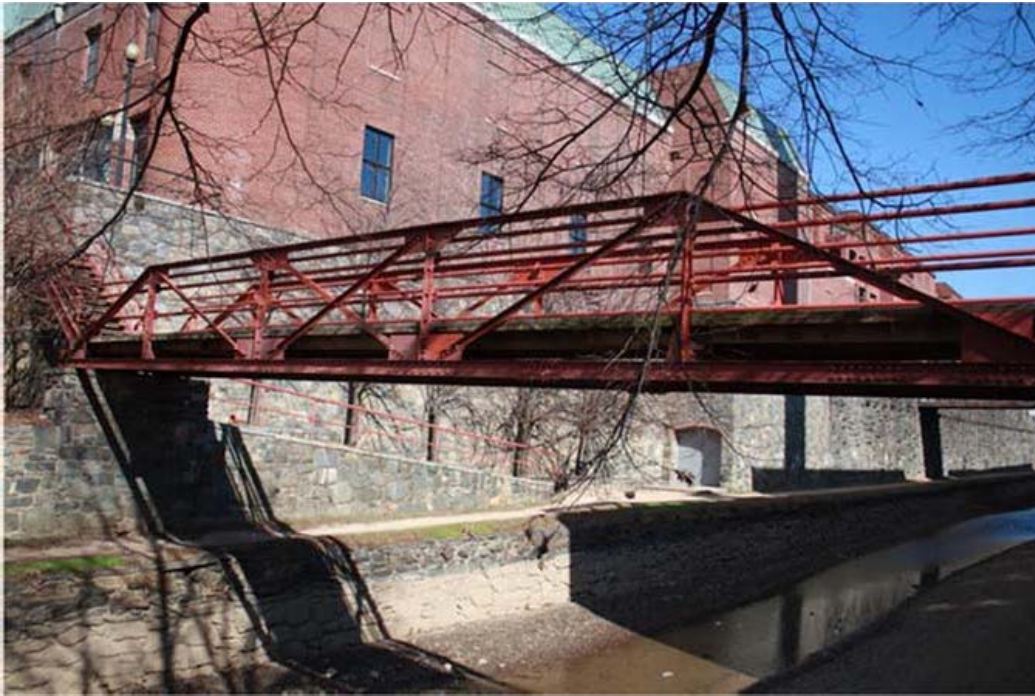
The Potomac Street Bridge. Originally, the bridge was wooden and part of the set of bridge constructed in 1831. (NCR CLP 2017).
