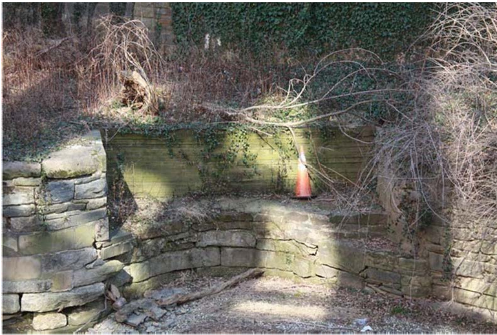
The side pond inlet located on the south corner of the Lock No. 1 prism. (NCR CLP 2016)
