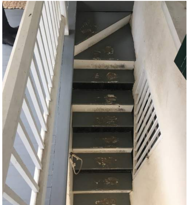
Figure 178: Non code and ABAAS complaint stair at east porch (BBB 2019)
