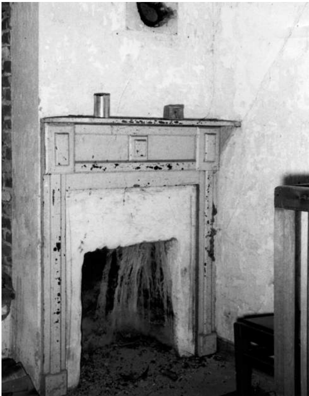
Figure 60: North Wing, Second Floor Before Renovation, Fireplace in Room 207 or 210 Looking Northeast, ca. 1950s. (CHOH NHP)
