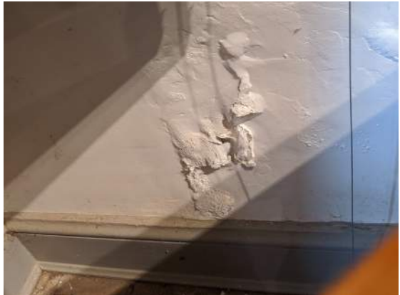
Figure 214: Plaster Delamination Below Chair Rail in North Wing, First Floor (BBB 2019)
