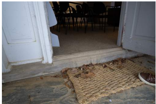
Figure 177: Six-inch step at Door 103A (BBB 2019)
