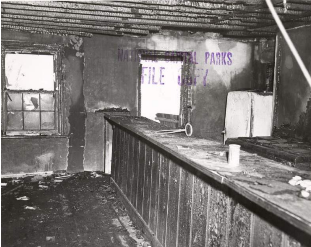
Figure 74: Fire Damage to South Wing Interior Looking Northwest, March 1954 (NPS)
