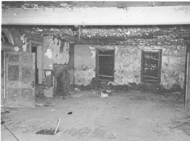
Figure 43: North Wing First Floor After Fire in 1948, looking NE. (NPS)
