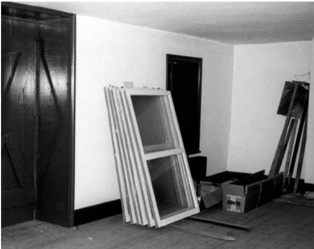
Figure 69: Center Section, Second Floor During Renovation, Southeast Corner Looking Southeast, ca. 1950s. (CHOH NHP)
