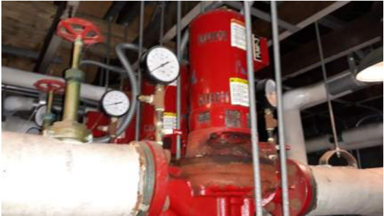
Figure 232: Heating Water Pumps (JPA 2019)
