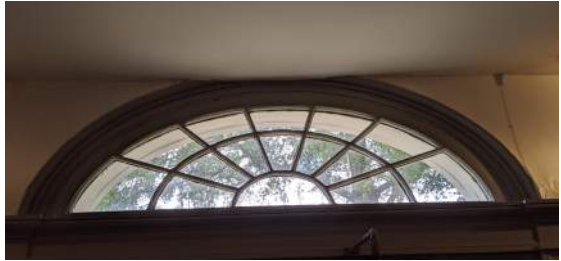
Figure 219: Bowed Ceiling at North Wall, First Floor North Wing (BBB 2019)
