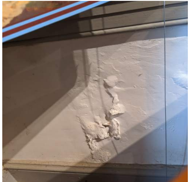
Figure 131: North Wing First Floor, Water Damaged Plaster at Northeast Corner (BBB 2019)
