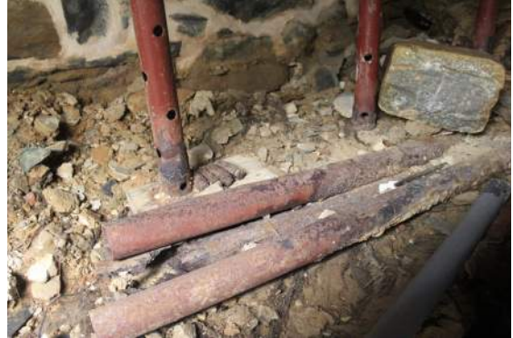
Figure 192: Corroded Shoring Posts at West Wall in Cellar of Center Section (Silman 2019)
