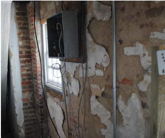
Figure 197: Mortar and Plaster Loss at Interior of North Wing Third floor, North Wall (BBB 2019)
