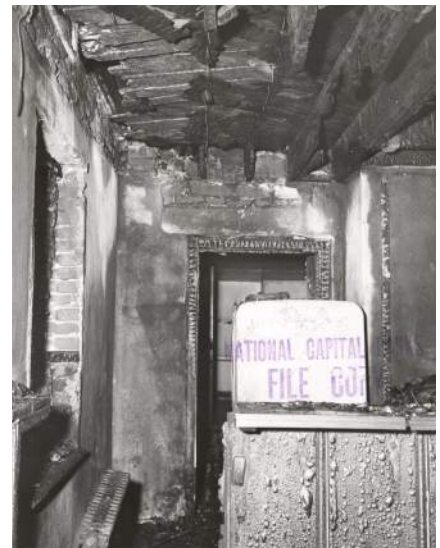
Figure 77: Fire Damage to South Wing Interior Looking North to Center Section, March 1954 (NPS)
