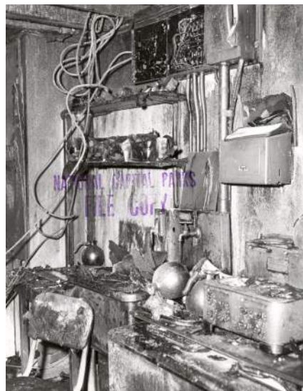
Figure 76: Fire Damage to South Wing Interior Looking Northwest, March 1954 (NPS)
