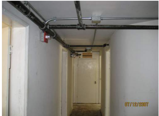
Figure 106: After Utility Installation, North Wing Second Floor, Looking East, Closet Still Present at East End, July 12, 2007. (NPS)
