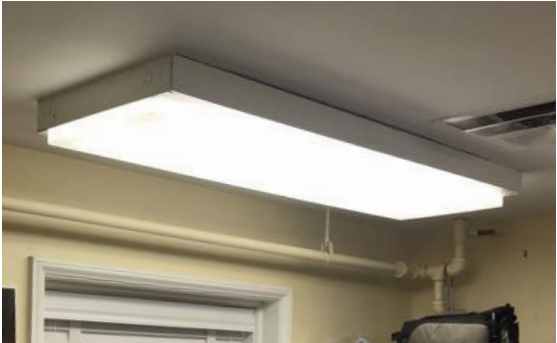
Figure 240: Architectural Office Lighting (JPA 2019)
