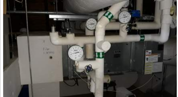
Figure 231: Typical Attic Fan Coil Unit (JPA 2019)
