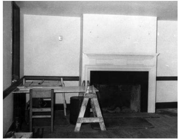
Figure 63: Center Section, First Floor During Renovation, North Wall Looking Northeast, ca. 1950s. (CHOH NHP)
