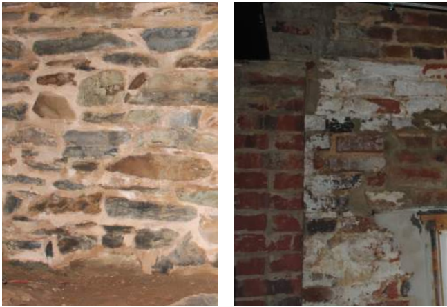
Figure 183: Original Stone in Cellar (L) and Brick in Third Floor (R) (BBB 2019)
