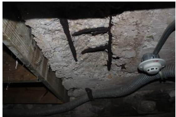
Figure 193: Concrete Slab in Poor Condition (Silman 2019)
