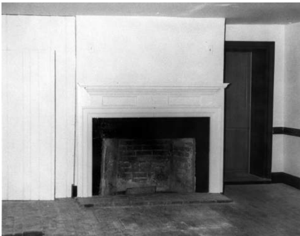
Figure 66: Center Section, First Floor During Renovation, South Wall Looking South, ca. 1950s. (CHOH NHP)
