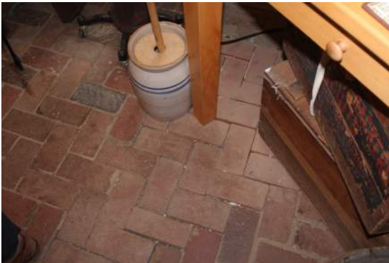
Figure 191: Brick Paving in North Wing Built over a Concrete Slab on Grade (Silman 2019)
