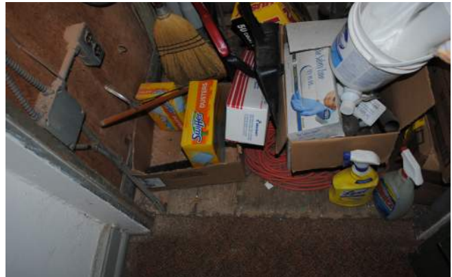
Figure 139: North Wing Second Floor, Wood Flooring in Closet Beneath Attic Stairs. (BBB 2019)
