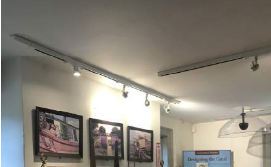
Figure 238: Track Lighting (JPA 2019)
