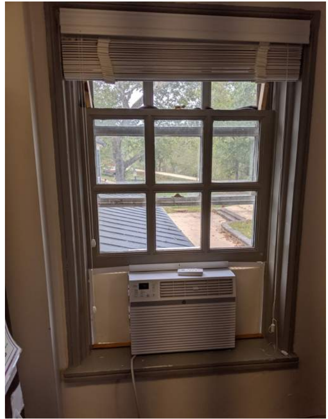
Figure 144: North Wing, Second Floor, South Window in Kitchen (Rm 211) Looking South (BBB 2019)
