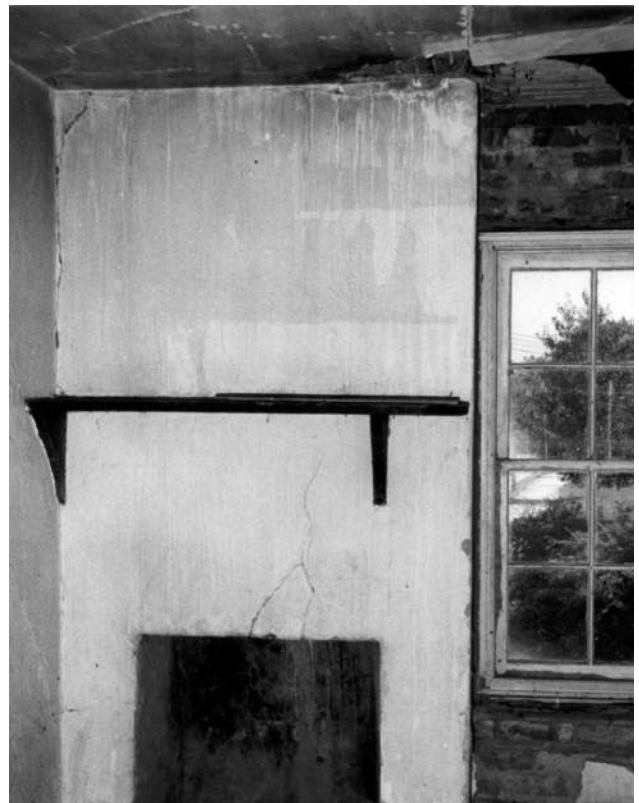
Figure 61: North Wing, Second Floor Before Renovation, Likely Fireplace in Room 209 Looking Northwest, ca. 1950s. (CHOH NHP)
