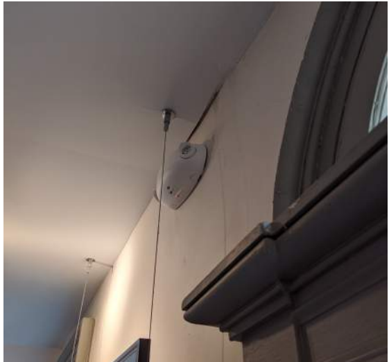
Figure 220: Sagging Ceiling at North Wall, First Floor North Wing (BBB 2019)
