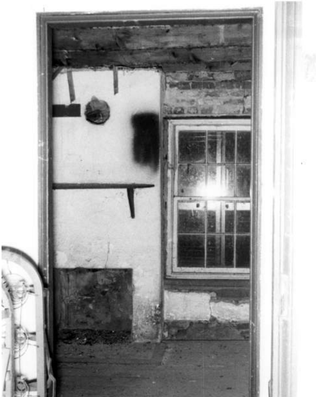
Figure 58: North Wing, Second Floor Before Renovation, Likely Fireplace in Room 206 Looking Northwest, ca. 1950s. (CHOH NHP)
