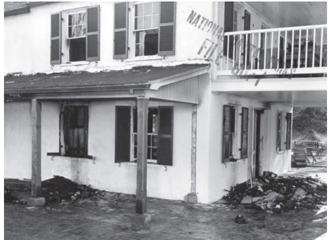
Figure 73: Fire Damage to South Wing Exterior Looking Northeast, March 1954 (NPS)
