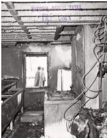
Figure 75: Fire Damage to South Wing Interior Looking West, March 1954 (NPS)
