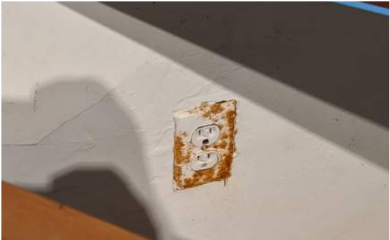
Figure 237: Corroded Receptacle in North Wing, First Floor (BBB 2019)
