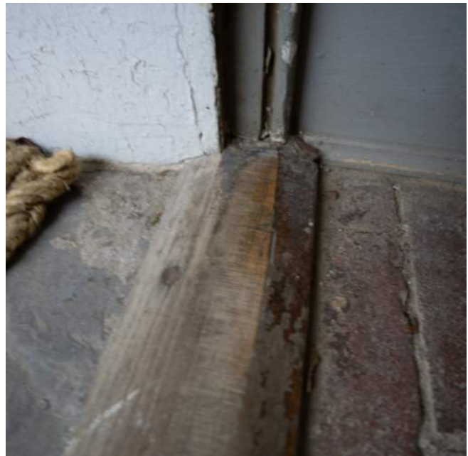
Figure 179: Non-ABAAS compliant threshold at Door 101B (BBB 2019)
