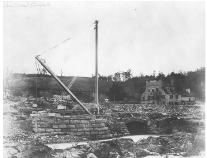
Figure 5: 1858 photograph taken during the construction of the intake dam, the Tavern appears in the background. (Library of Congress)
