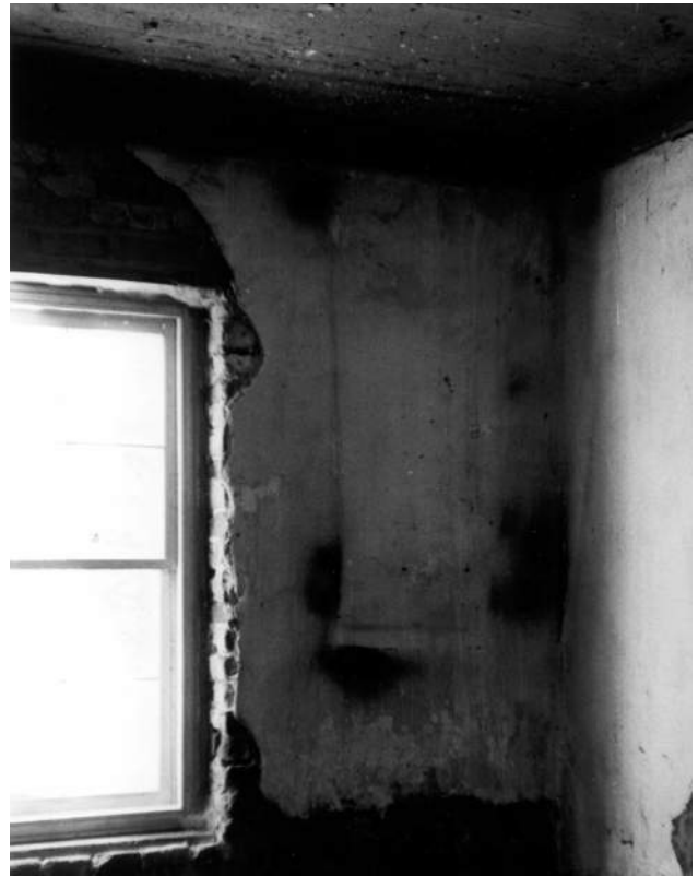
Figure 59: Likely North Wing, Second Floor Before Renovation, Unknown Room, ca. 1950s. (CHOH NHP)
