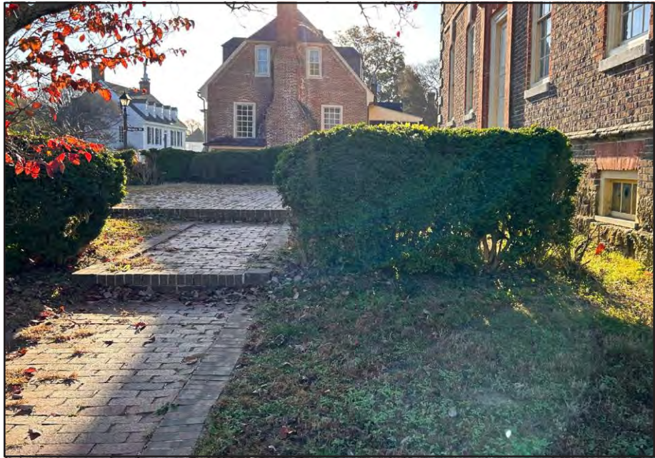
Figure 4.1 2023 photograph of the existing two steps in the walkway from the terrace to the front court.
