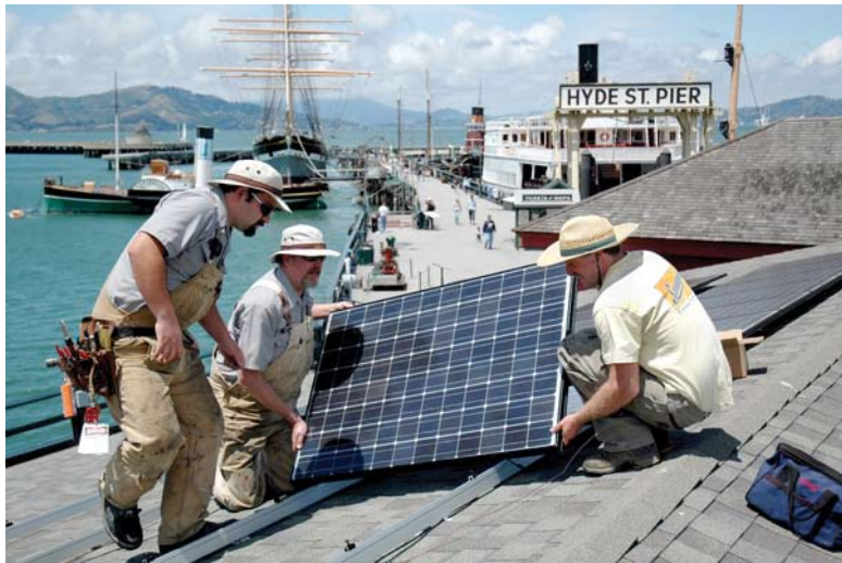
Photovoltaics power the boat shop, shipwright shop, and ranger office.
