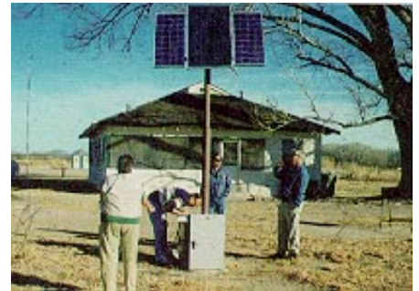
SAN PEDRO PROJECT OFFICE Sierra Vista, Arizona San Pedro Riparian National Conservation Area 200-watt array, 200-amp-hour battery provides power for host and lights for contact station building.
