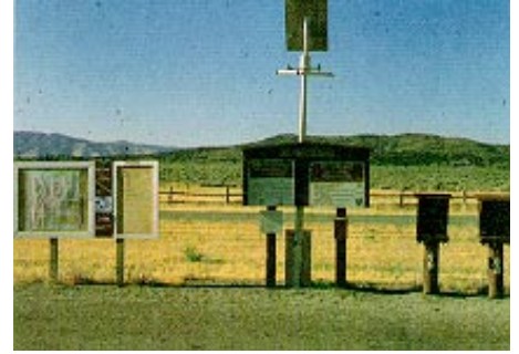
FILLMORE FIELD OFFICE, UTAH Little Sahara Recreation Area 50-watt array, 200-amp-hr battery provides lighting for fee station at night.
