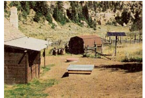
VERNAL FIELD OFFICE, UTAH Jarman's South Camp Cabin Provides power for lights, small appliances, and water booster pump at this administrative site.
