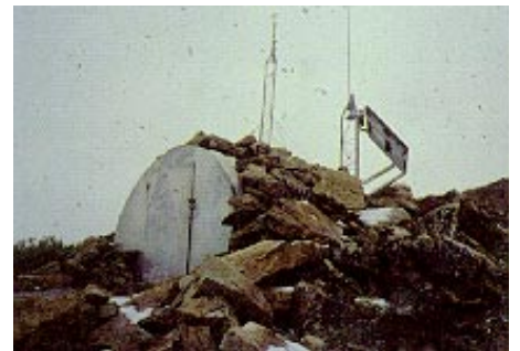
WINNEMUCCA DISTRICT, NEVADA Granite Peak 80-watt array provides years around communications in remote district areas.
