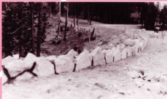
Mason dressing stone to be incorporated within a guard wall near Pumice Point, 1934.
