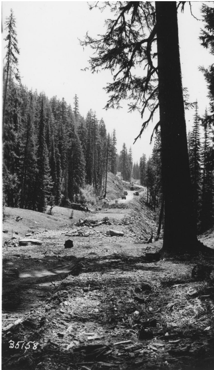
History #7: Rim Drive road construction east of the Castle Crest Wildflower Trail, 1939 (Struble, BPR).
