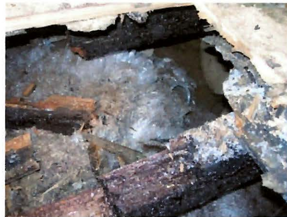
Rotten floor joists from freeze and thaw of moisture in crawlspace
