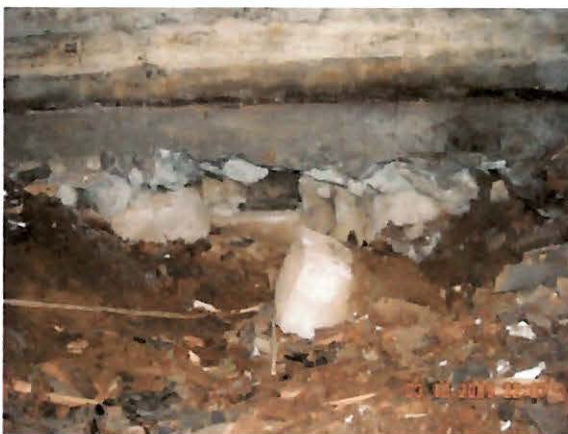
Deteriorated masonry foundation
