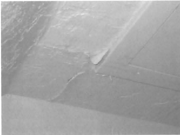
Cracked and spalling plaster on ceiling
