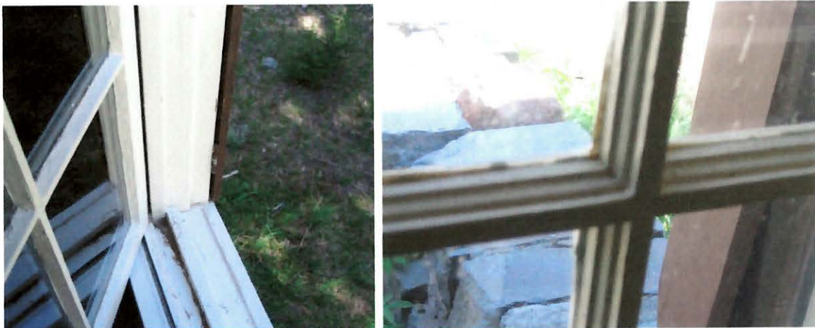
The window frame is composed of several members and all details should be carefully noted and reproduced if windows are rebuilt
