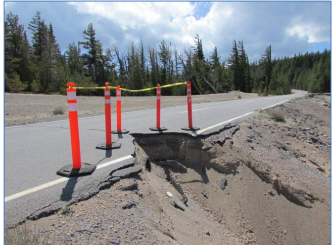
Figure 5. East Rim Drive at Grotto Cove prior to emergency stabilization and repair in 2014. Photo by Jen Beck.
