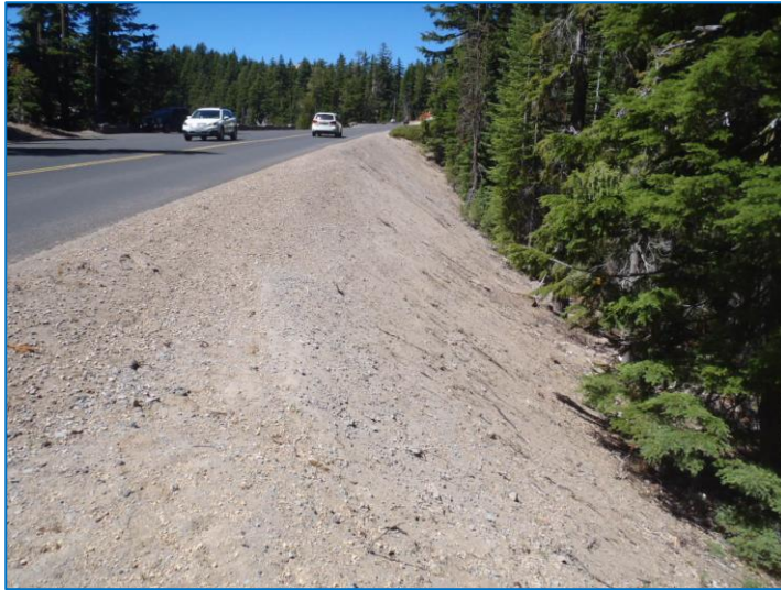
Figure 17. Deep patch operations along East Rim Drive required unanticipated disturbance of areas including this slope. Photo by Carrie Wyler.
