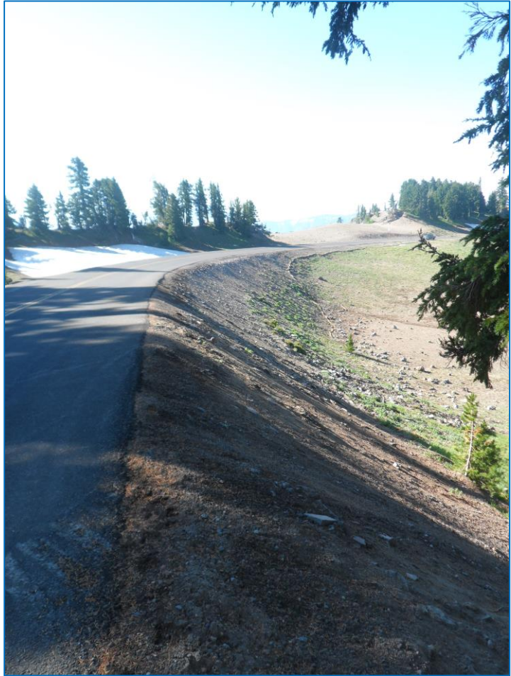
Figure 17. Deep patch operations along East Rim Drive created unanticipated disturbance of areas including this slope. Photo by Carrie Wyler.
