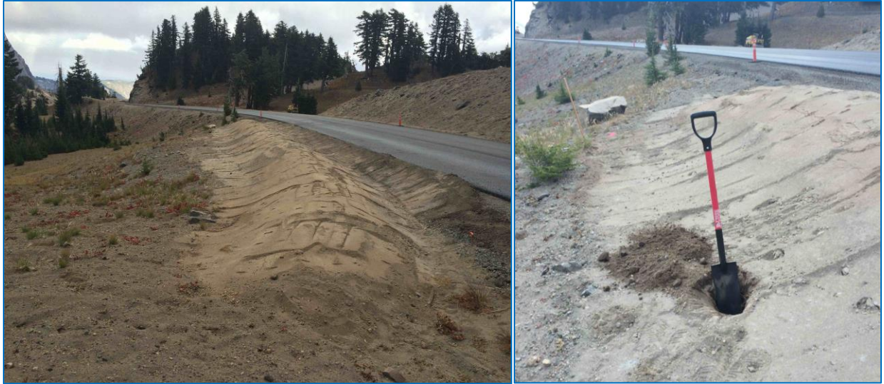
Figure 19. An obliterated pullout with insufficient site preparation, as the restored area looks more like a “worm” of placed topsoil rather than a natural landscape feature (left). Obliterated pullouts were inspected for signs of soil compaction (right). Photos by Ken Stella.
