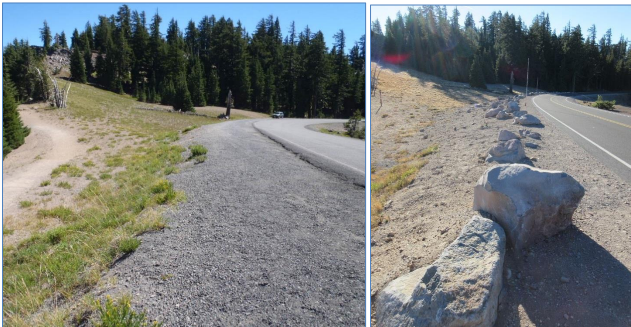
Figure 1. User-created pullout before (left; photo by Jen Hooke) and after (right; photo by Tara Chizinski) obliteration as part of the Rim Drive Rehabilitation project.
