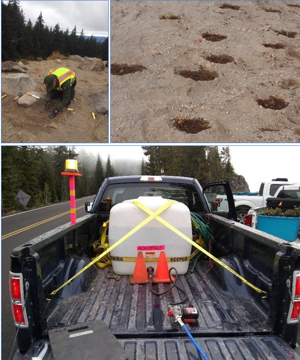
Figure 12. Upper left: Building a berm for a plant. Upper right: Recently installed plants with compost and soil berms to contain water. Photos by Tara Chizinski. Bottom: Truck-mounted water tank used to water newly planted and mulched plants. Photo by Carrie Wyler.
