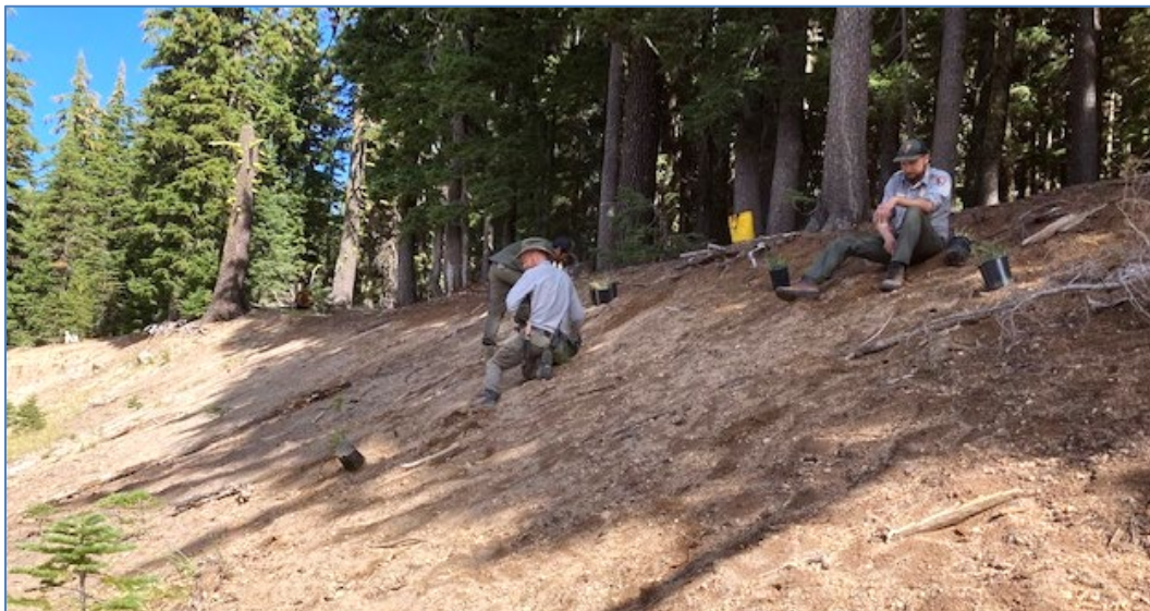
Figure 13. Planting the steep and difficult to restore eastern embankment at Cleetwood Cove parking lot. Photo by Carrie Wyler.
