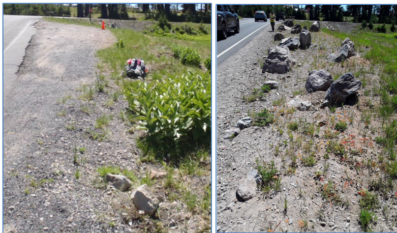
Figure 11. User-created pullout (restoration site SWRD1) before (left) and after (right) rehabilitation and revegetation efforts. Photos by Carrie Wyler.
