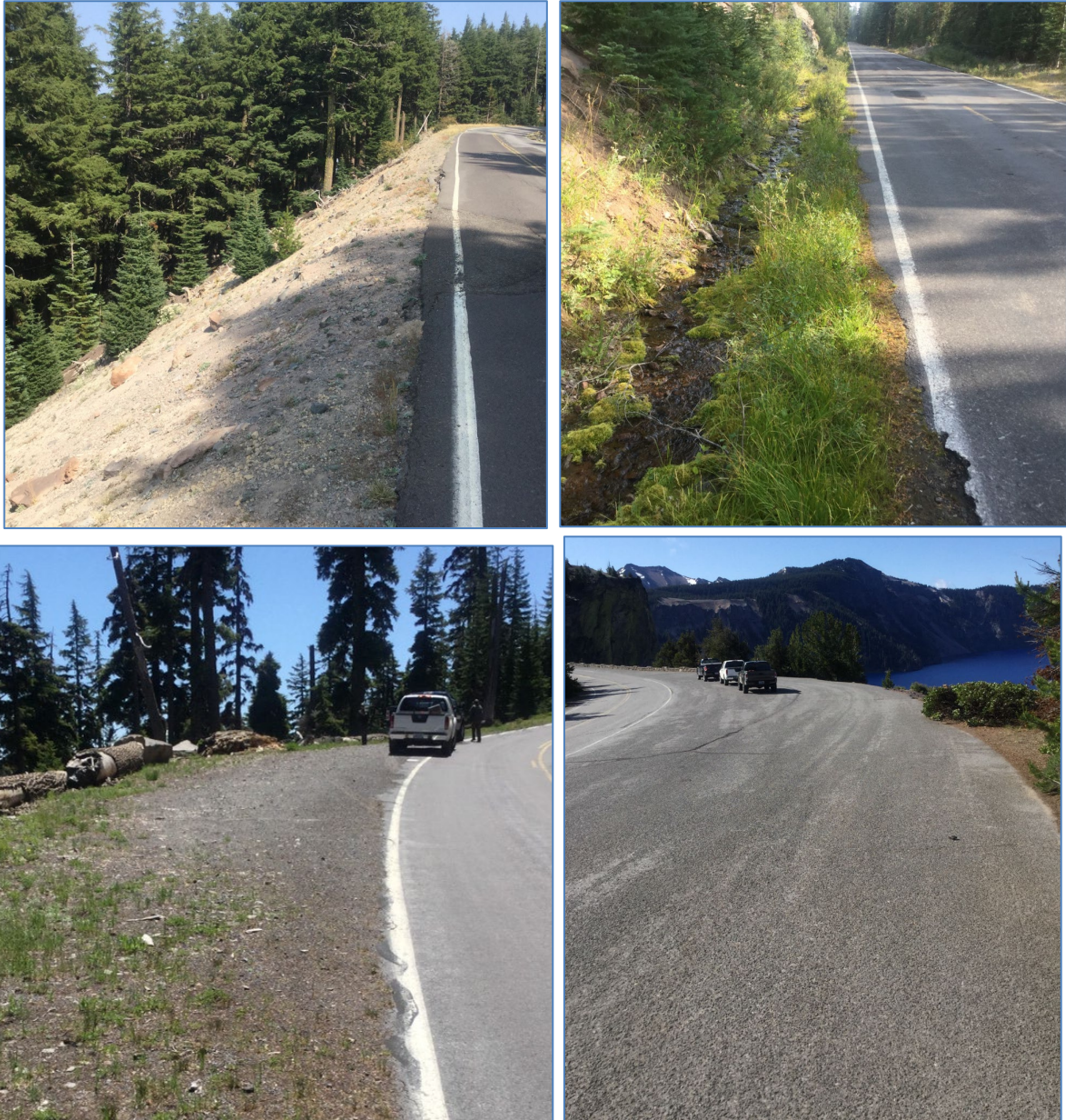
Figure 1. Top: Example of a deep patch area (left). Road stabilization section that will destroy a unique roadside riparian area as part of the Rim Drive Rehabilitation project (right). Bottom: User-created pullout (left). Example of an excessively wide pullout within the project area (right). Photos by Scott Heisler.
