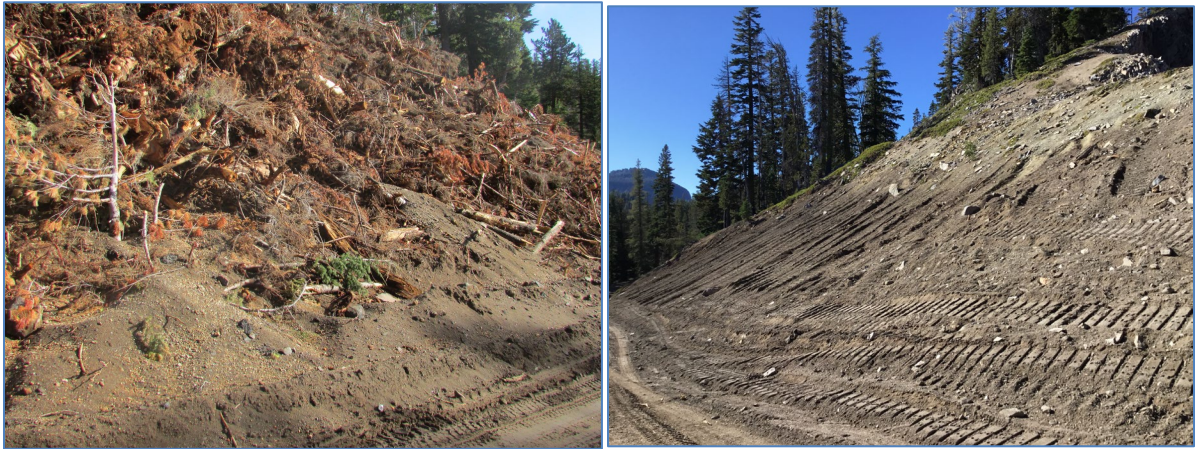
Figure 22. Slope disturbed at Roundtop Quarry by slash piling and ground disturbance in 2015 (left); same slope after removing slash and recontouring in 2018 (right). Photos by Jen Hooke.
