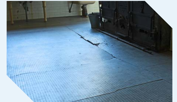
Failing kitchen floor at Plum Orchard.
