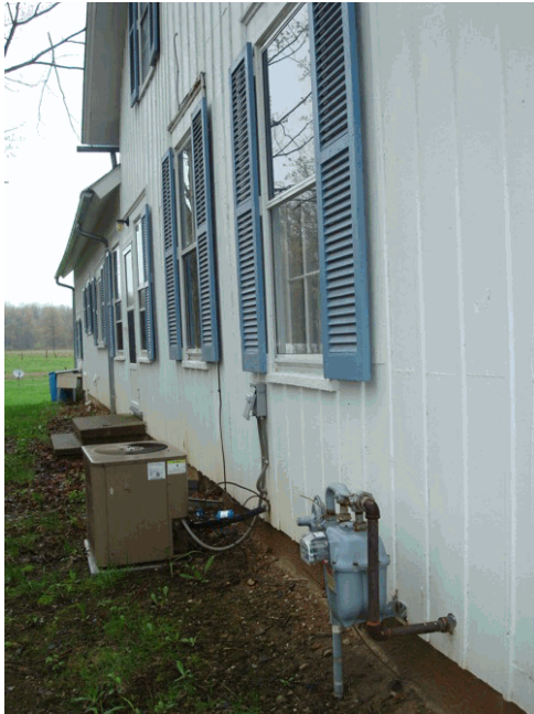
Image of modern electrical and HVAC systems next to the house (Jackson 2011)
