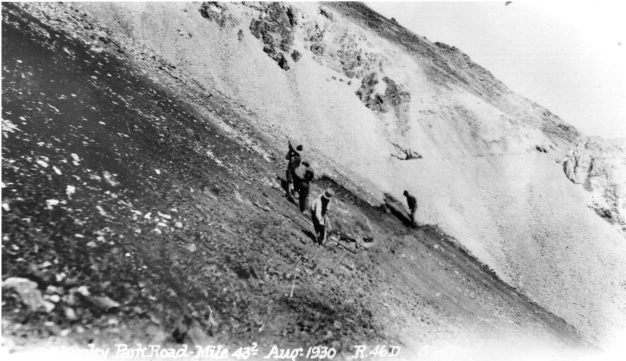
Building the High Line route (Alaska State Library, Alaska Road Commission Collection, 61-2-230)
