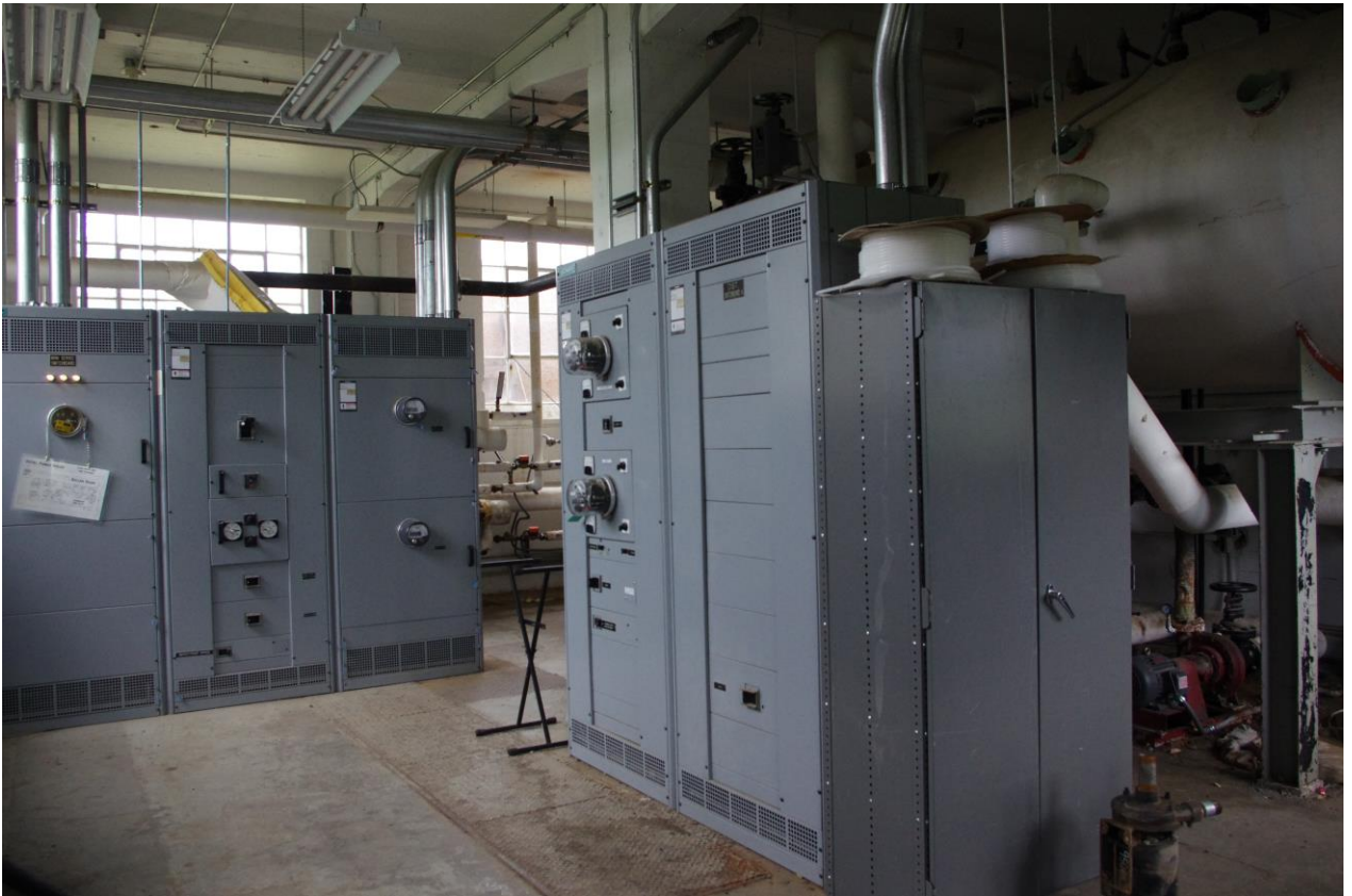
12 of 15. The Power House, interior, electrical room, looking south.
