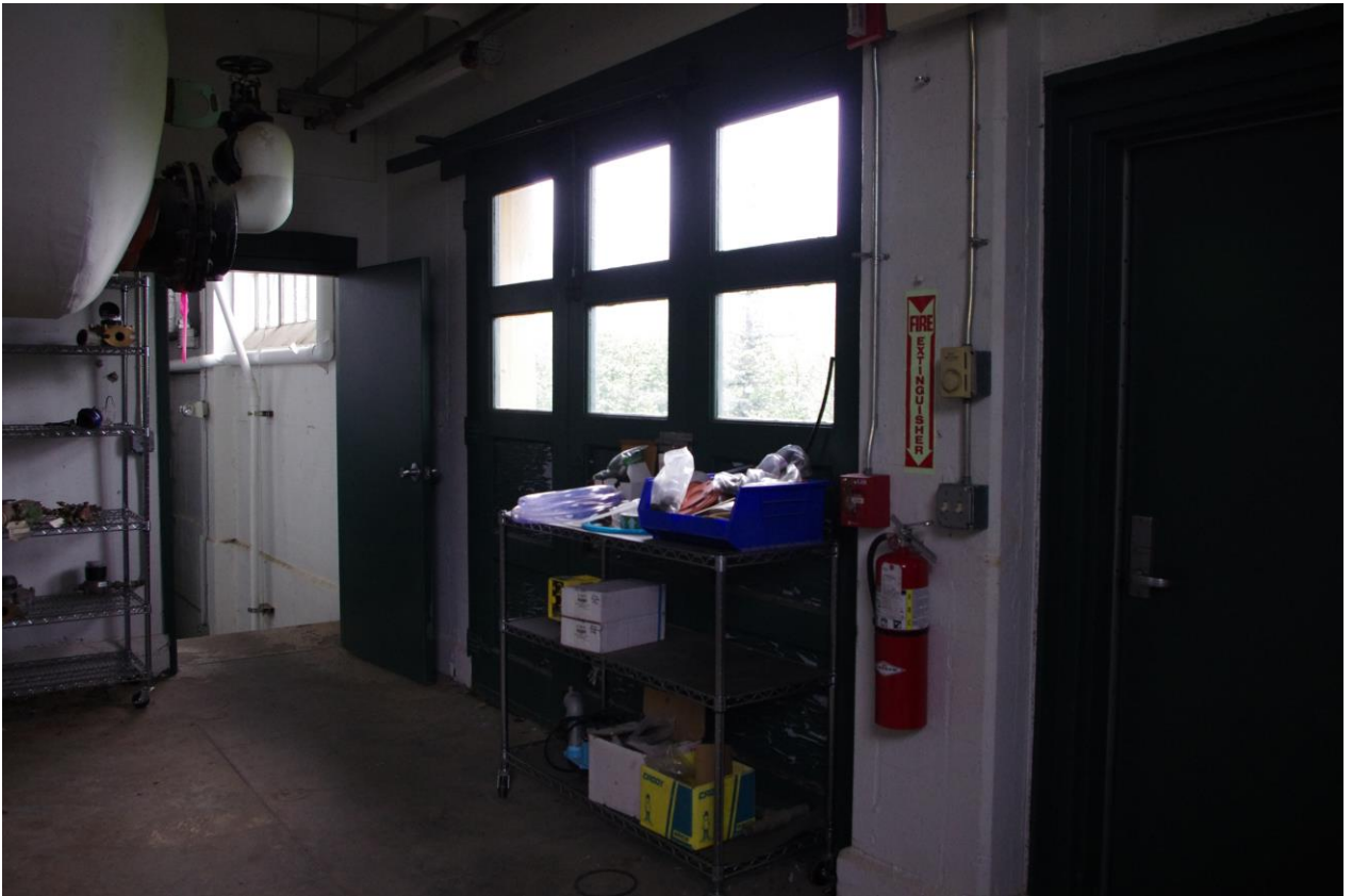
14 of 15. The Power House, interior, electrical room, looking north.
