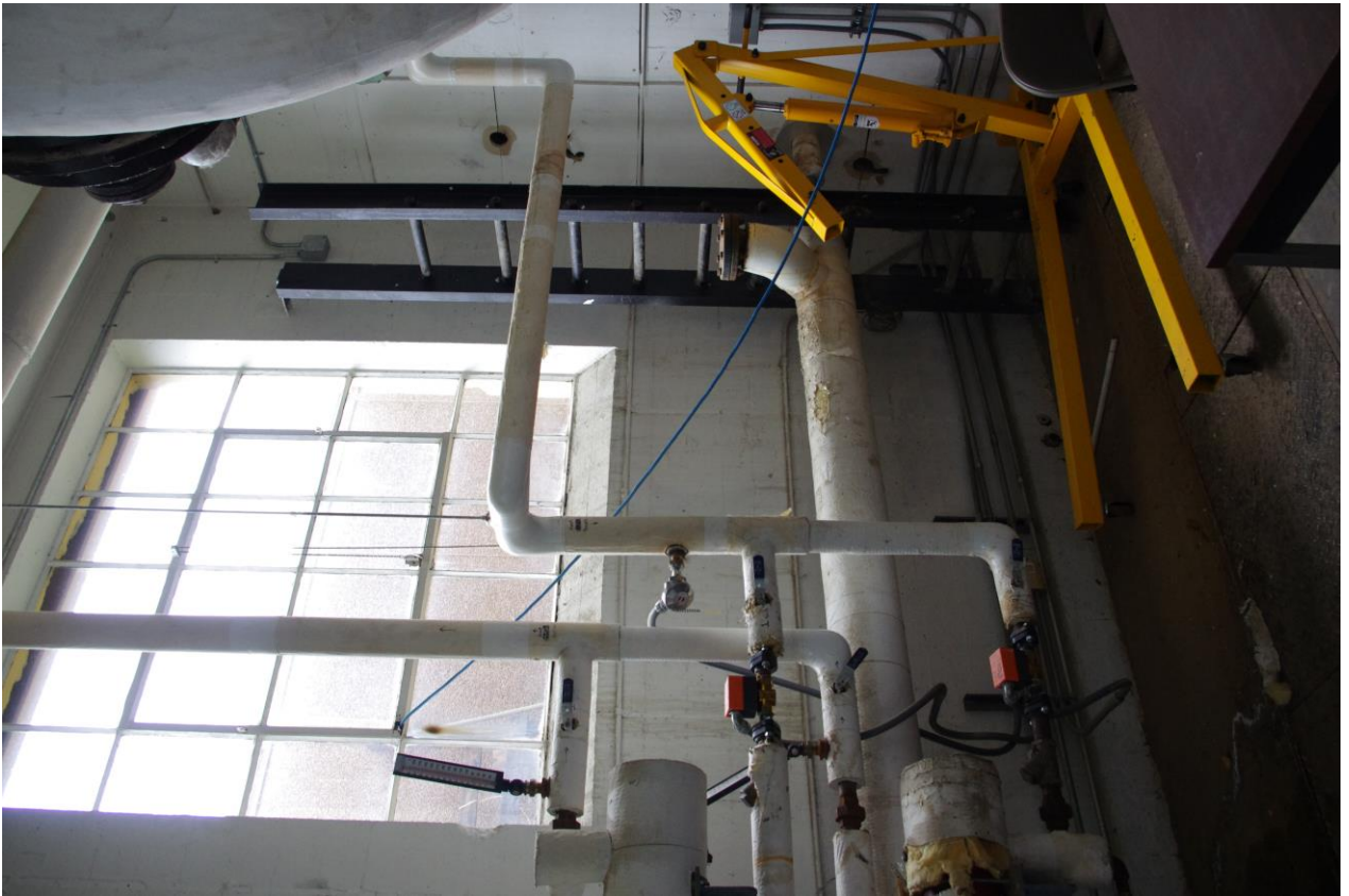
13 of 15. The Power House, interior, electrical room, looking southwest.
