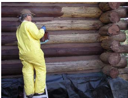
Restoration work on historic log buildings, a project funded by the fee demonstration program.
