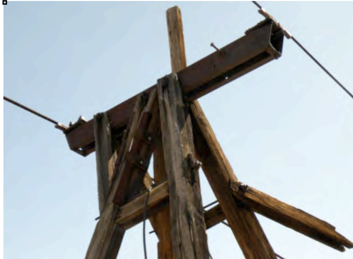
Figure 1. Top of tower 6, showing dangling southwest saddle beam brace. Photo: UVM School of Engineering
