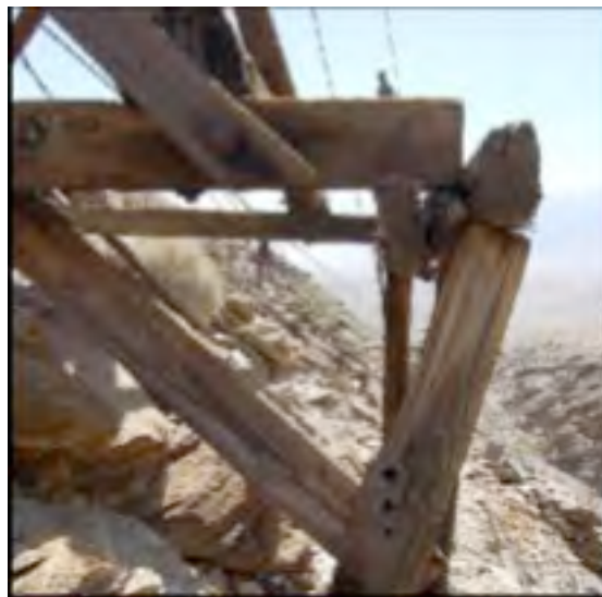
Figure 3. Tower 8, northwest corner of secondary frame showing failure. Photo: UVM School of Engineering
