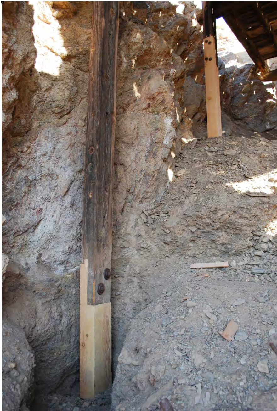
Figure 6. Column repairs at D8 (left) and D7 (right) at the Lower Terminal.
