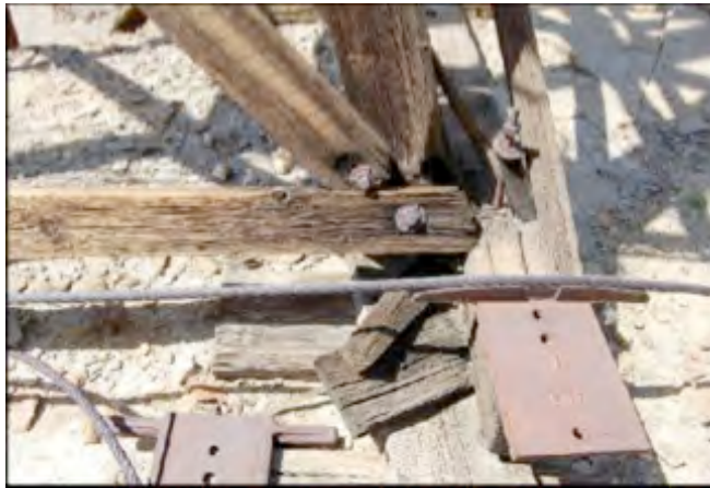
Figure 2. Tower 8, northeast column, shown fallen from its sill. Photo: UVM School of Engineering
