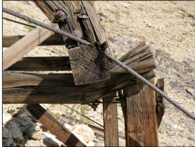
Figure 4. Failure of west secondary sill, tower 9. Photo: UVM School of Engineering
