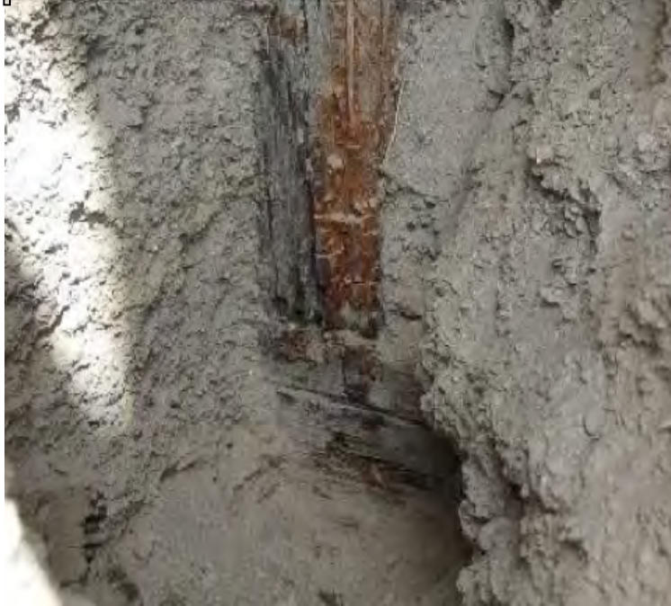
Figure 5. Base of column D8 prior to treatment, buried and severely decayed.
