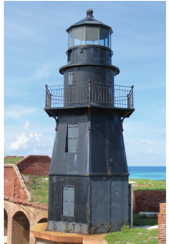
1876 Lighthouse with Corrosion
