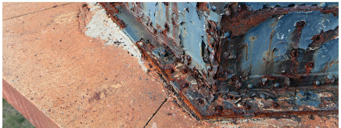
Corrosion at Base of Lighthouse
