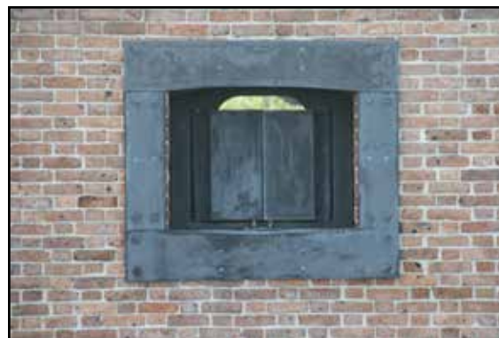
Replicated Totten Shutter assembly embedded in scarp wall with shutter doors and an exterior breast plate
