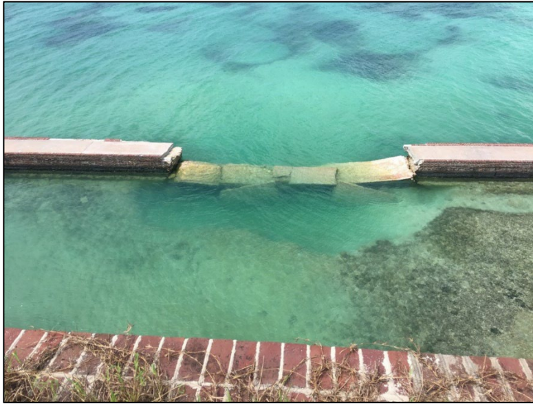
Fig 35. Hurricane damage to counterscarp (Photograph provided by Glenn Simpson, DRTO Park Manager).
