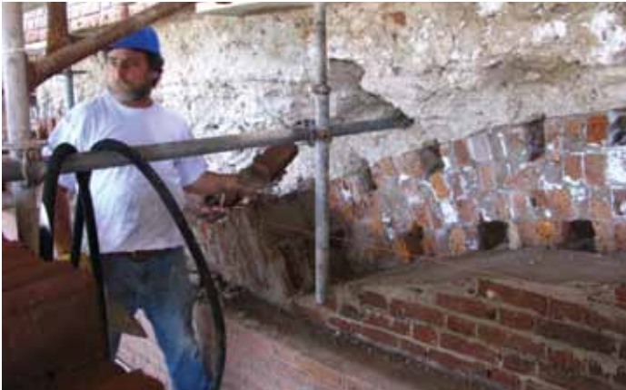
Figure 9: Tie bricks let into the undamaged vaulting tie the new vaulting into the old. The coral concrete is seen above.
