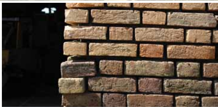
Figure 5: Mortar loss is severe in many areas.
