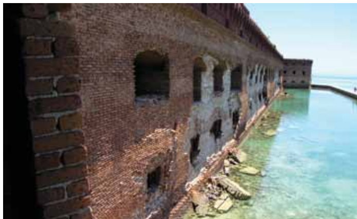
Figure 7: The damage to several fronts is severe but none as bad as that on Front 3.
