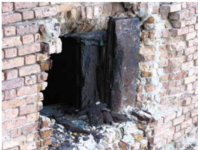
Figure 6: Corrosion of the embedded iron Totten shutters has severely damaged the masonry surrounding the embrasure openings.
