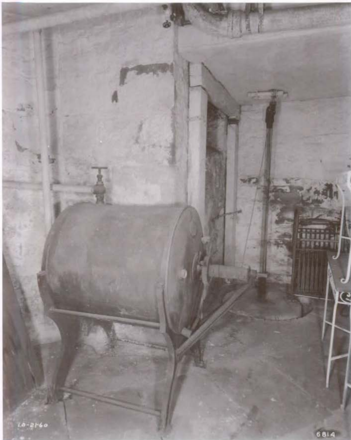
Figure 37. Room B9, northeast corner, showing the obsolete Springfield Gas Machine, 1960.
