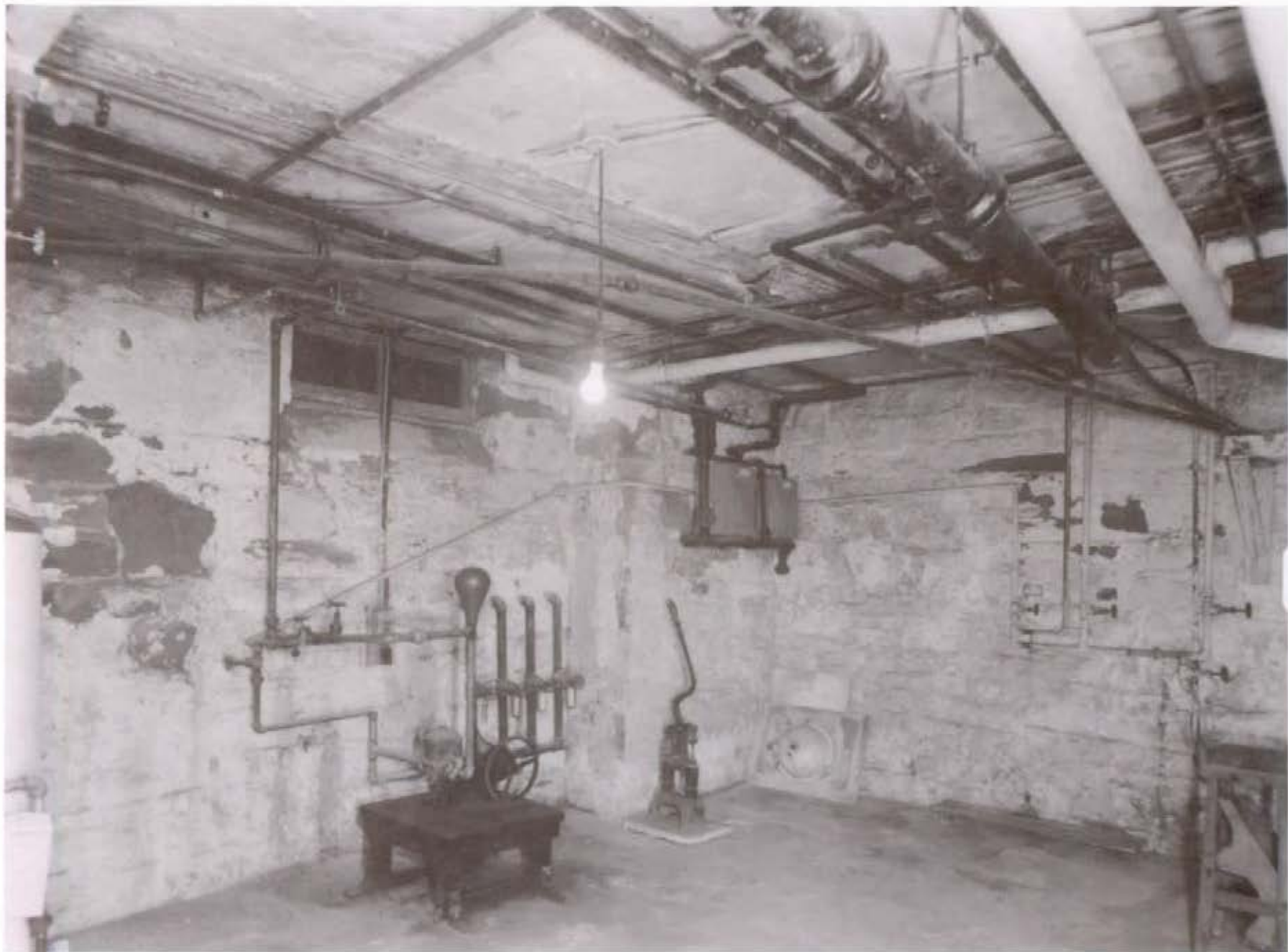
Figure 39. Pump Room (Room B14), northwest tower, showing the cistern valves and water pumps, 1960.
