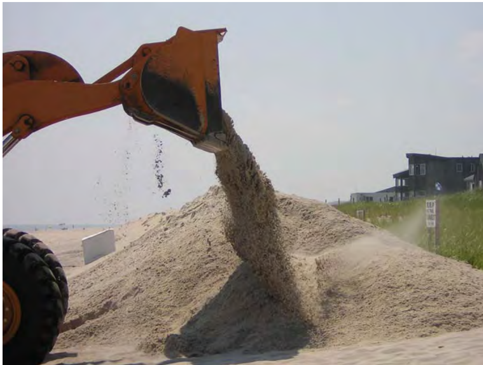
Figure 3. Photos showing stages of the beach scraping process taken on July 31, 2007 at Kismet, Fire Island. Sand is pushed into shore-perpendicular ridges (top), then dumped in front of the existing dune to create an anthropogenic foredune (bottom). Top photo: Erika Lentz. Bottom photo: Meredith Kratzmann.
