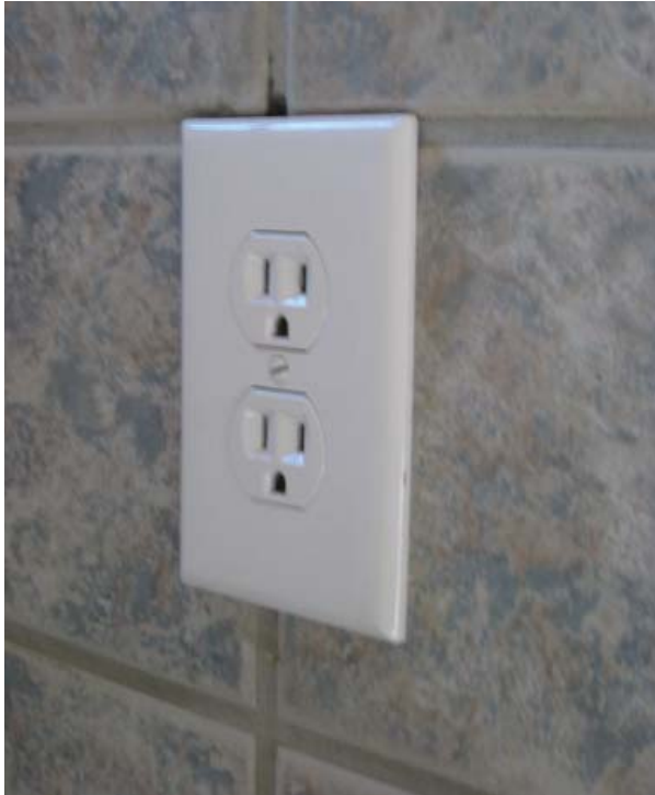
Figure 126. Typical outlet cover.
