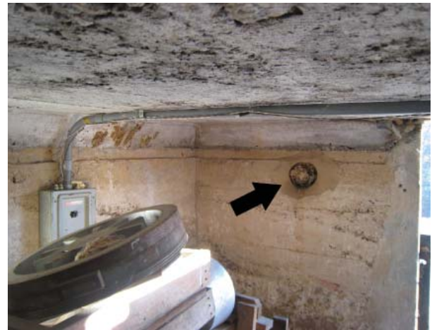
Figure 72. Southeast oblique. Note 8" diameter opening in south exterior wall.
