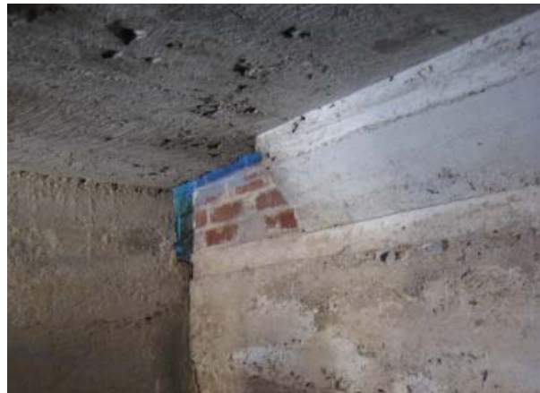
Figure 75. Slot in northwest corner of 1931 ceiling slab allows carriage door to slide open.
