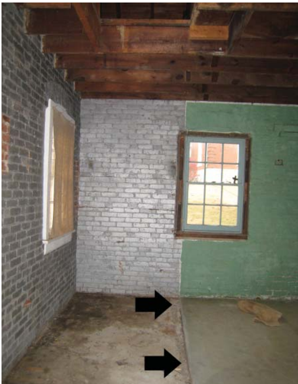
Figure 91. North wall of west section. Note imprint of wall enclosing ladder stair and hatch above.
