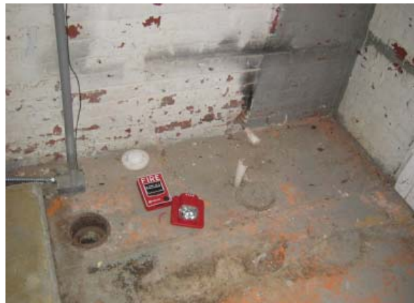
Figure 54. Remnants of plumbing lines and drains at southwest corner of first floor.
