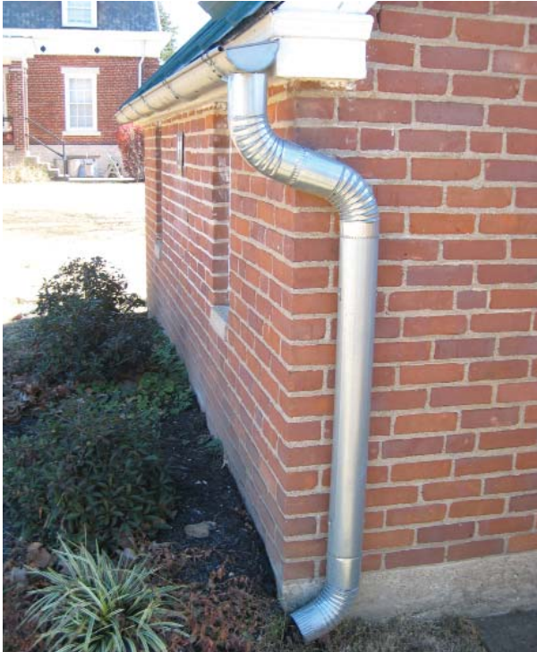
Figure 130. Round downspouts take rainwater to grade.
