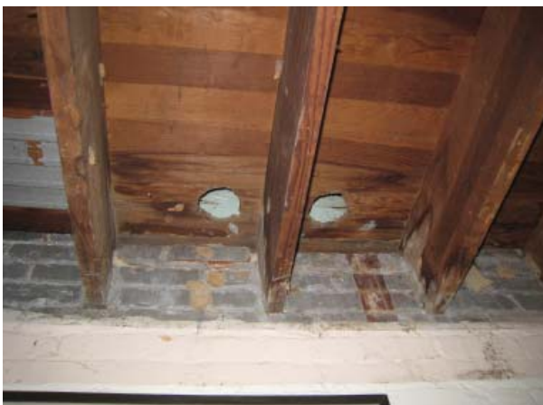
Figure 82. Two 4" diameter holes in loft flooring. Note water stains on flooring which may have come from a cistern or leaks from the adjacent loft doorway.
