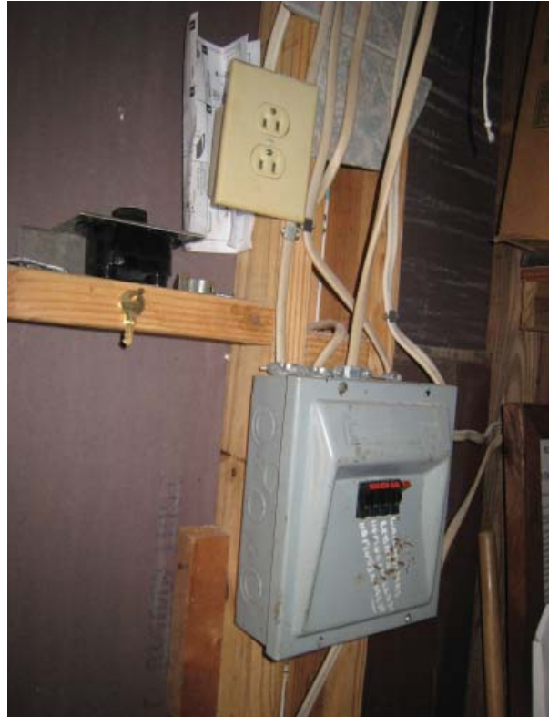
Figure 124. Electrical panel in Service Closet.
