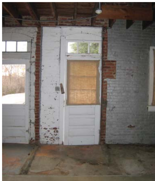
Figure 18. 2010 View looking west showing location of former bathroom partitions. Original doorway is on the left, window converted to doorway is in the center; original window is on the right. Opening to the loft is visible at the upper right.
