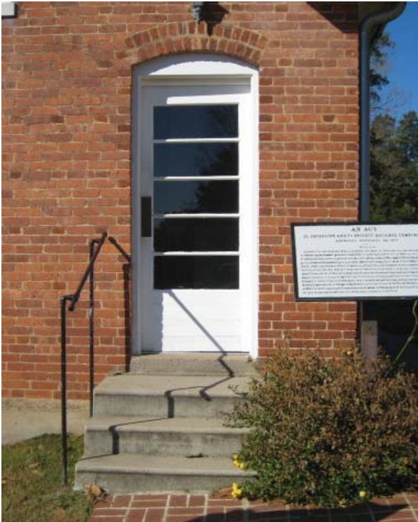
Figure 64. Original doorway at first-floor east elevation. Transom and door were removed when floor raised in 1931.
