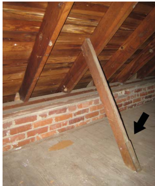
Figure 47. Rafters have bird's-mouth joint at wall plate. Diagonal tie-down bracing between rafters and floor joists with metal strap to attach to joist.
