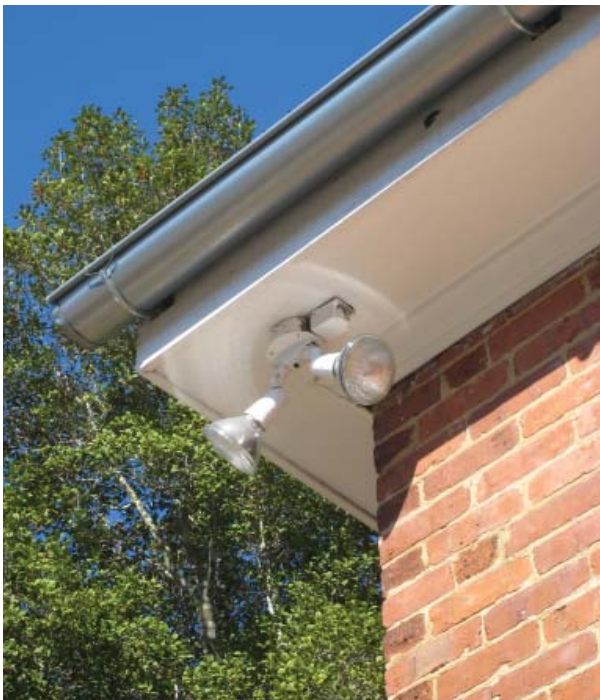
Figure 52. Floodlights at stone steps.
