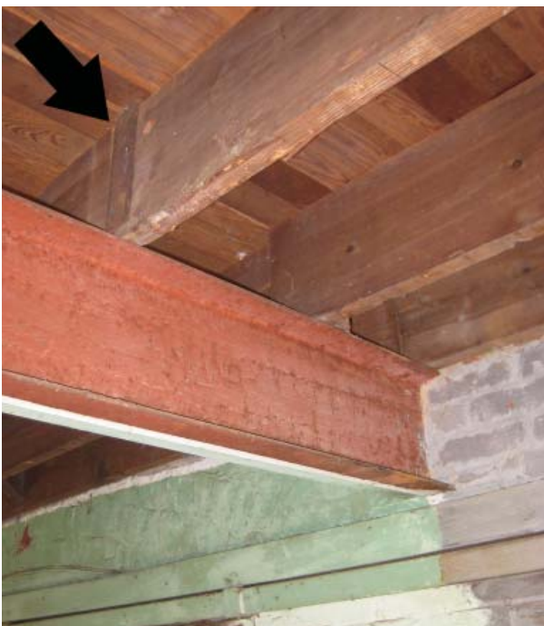
Figure 49. Rafter tie-down strap attached to joist spanning from steel I-beam girder to perimeter wall.
