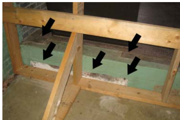
Figure 90. Ghostmarks for previous step to doorway atop raised concrete floor of Section 101.
