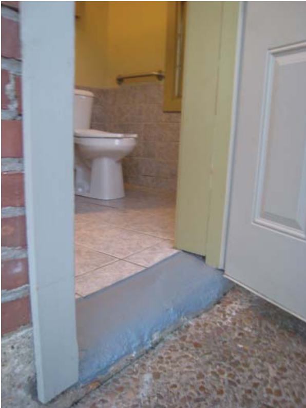
Figure 134. Entrance platform is 4" lower than restroom floor level.
