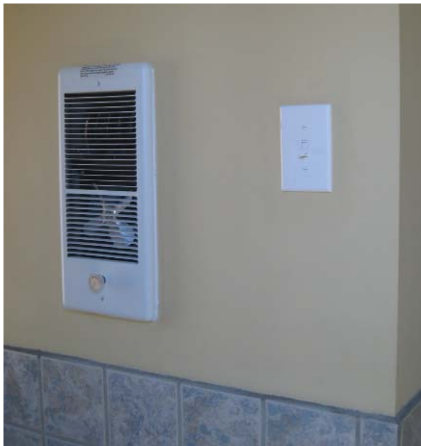
Figure 123. Typical wall heater and switch plate.
