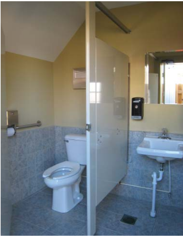
Figure 140. West wall with toilet enclosure in south section and lavatory in center section.
