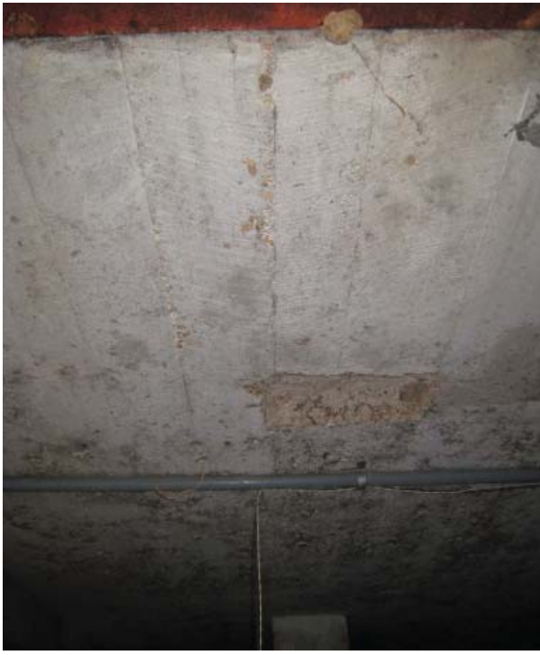
Figure 73. Wood-form indentations on underside of ceiling slab.
