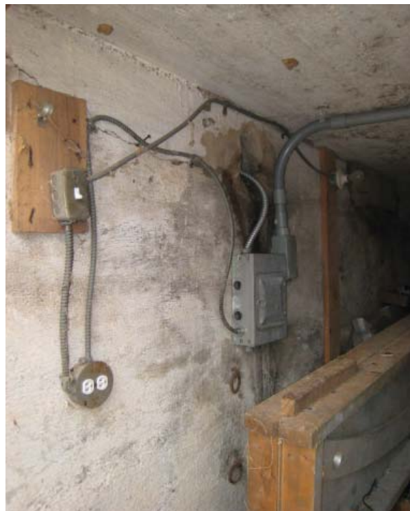
Figure 50. Electrical panel and wiring in basement Room 001.
