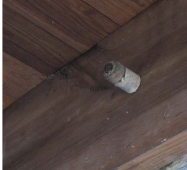
Figure 53. Rare surviving ceramic knob for early electrical wiring.
