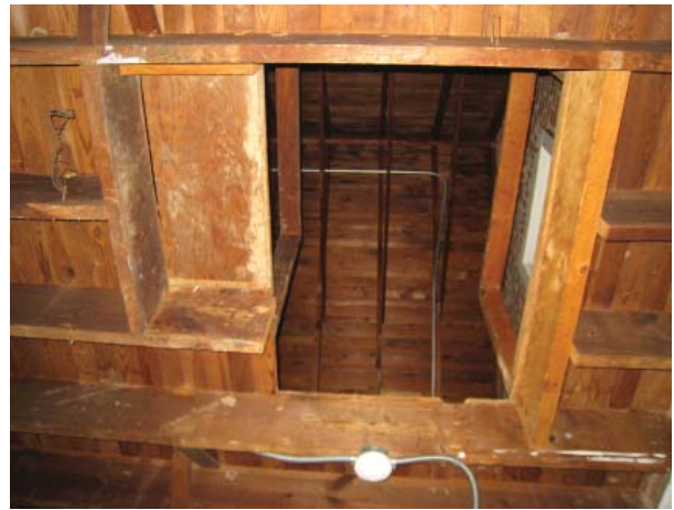
Figure 95. Original opening for ladder access to loft with later modifications. Note patch partially enclosing original opening. (See Appendix A Sheet 4)
