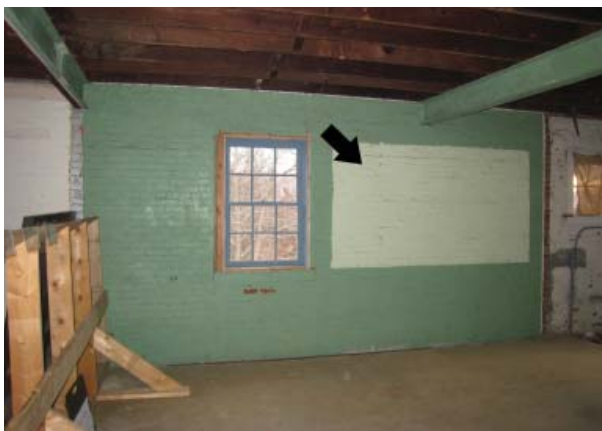
Figure 89. South wall of center section. Area of light colored paint was behind a display board when the room was repainted.
