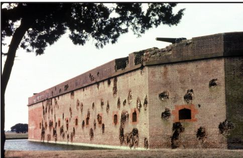
The damaged walls of Fort Pulaski are visible from the Fort Perimeter Trail.
