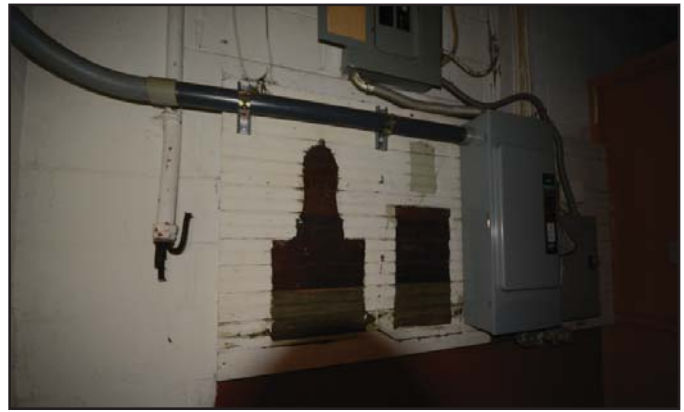
Figure 30: Electrical panels in rear of 1029 Gurnee Avenue. Photo by author, 2020.
