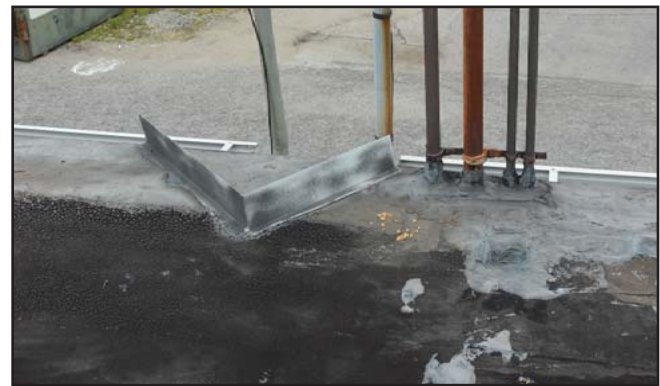
Figure 21: A roof cricket at rear of building between 1029 and 1025 Gurnee Avenue roofs divides water flow between the two building's gutters. Photo by author, 2020.
