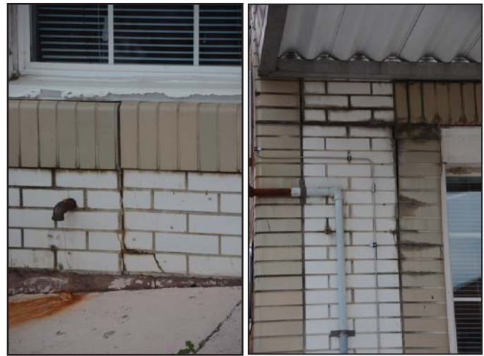
Figure 14: Cracking and water staining in the white and tan brick veneer on the east elevation. Left is below the Gurnee Avenue-facing window and right is left of the same window's header. Photo by author, 2020.
