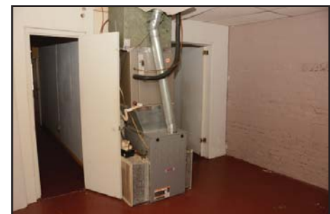
Figure 28: HVAC mechanical unit on the east side of the historic partition. Photo by author, 2020.
