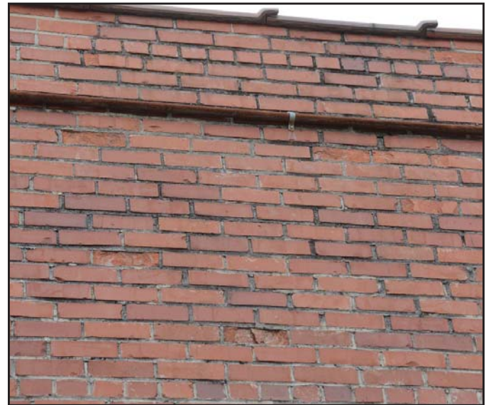
Figure 15: Some brick face spalling and wetness is evident on the upper portion of the north elevation. Photo by author, 2020.
