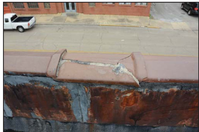
Figure 22: Terra cotta coping tiles. The center tile in this image is cracked and has been repaired with mortar. Photo by author, 2020.
