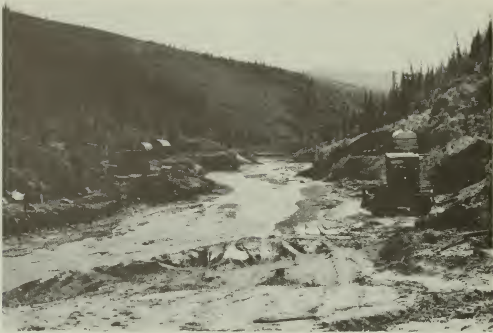
Illustration 13. Channel disturbance associated with placer mining on Mascot Creek. Note unbermed fuel and chemical storage tanks adjacent to Mascot Creek. Also note access road across tundra slope in background, with large slump at bottom.
