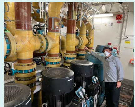
An NPS Scientist inspects the emission gas cleaning system ('scrubber') installed on a cruise ship operating in Glacier Bay.
