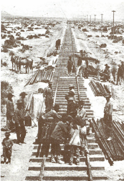
Railroad construction was labor intensive, with each worker assigned a specific job.
