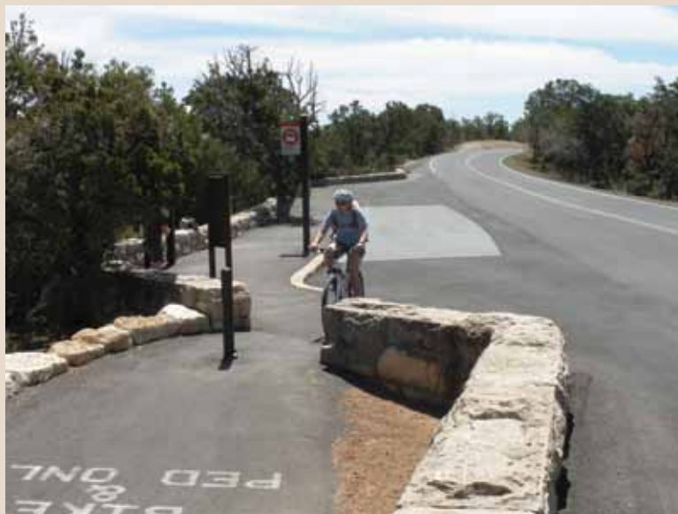
The new portion of the accessible Hermits Road Trail, which is used as a combination hike/bike trail. NPS photo
