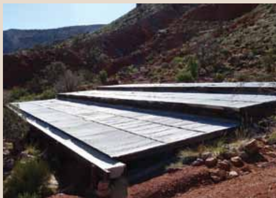
Water catchment system at Tuweep that provides potable water for residence. NPS photo
