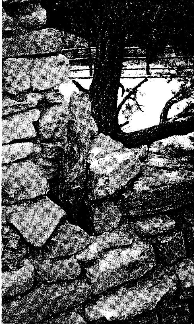
Figure 14. This image illustrates the tree well on the west side of the building, though the tree is no longer extant. Maier, ever sensitive to the surrounding landscape, incorporated this unplanned feature into the building during construction to accommodate an existing tree rather than cut it down. Photo dated May, 2000.
