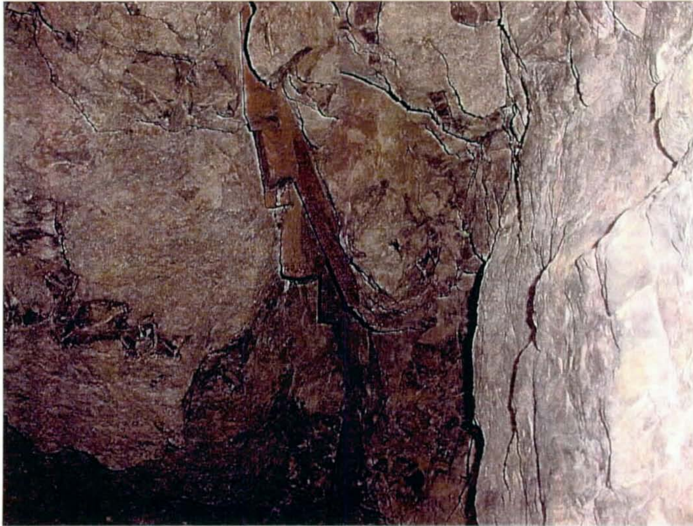
BASEMENT, SHOWING CONTINUING CRACK AND WOODEN WEDGES
