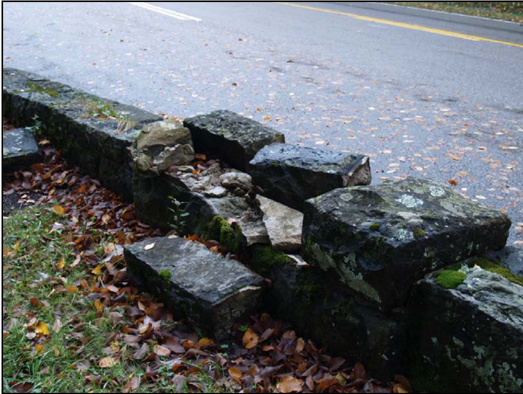
Figure 39. Damaged Masonry Guard Wall at Pull Off.
