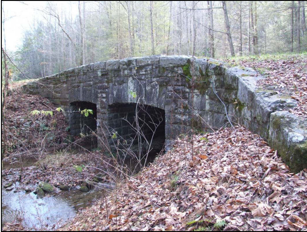
Figure 32. Structure 1.10, Double Box Culvert with Stone Masonry-Faced Headwall and Parapet, Milepost 2 (No. 22).
