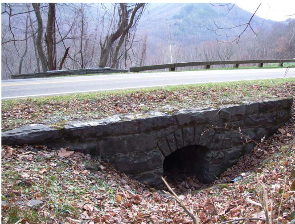
Figure 35. Structure No. 3.90, View of west headwall, looking east towards east headwall capped with stone parapet/guard wall.
