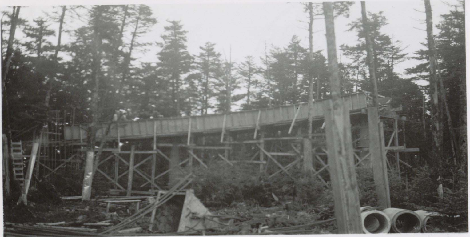
Fig. 6 "Portion of Ramp Showing Forms and Supports" Showing the proximity of trees to the ramp and the protective casings given to several trees. NPS photograph by R.A. Wilhelm, 1959. Archives of GRSM.
