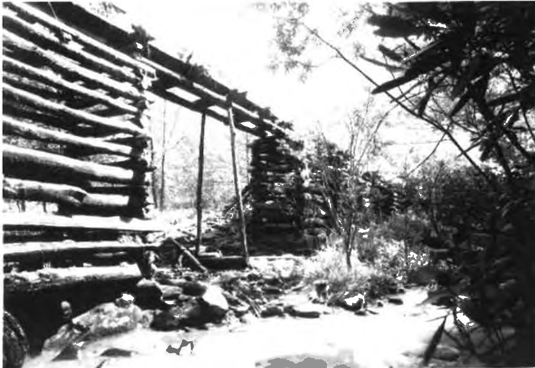
Figure 3. May 1937 photograph of Flume prior to repair, looking west (upstream) toward Mill Race (NPS Neg. No. 3087)
