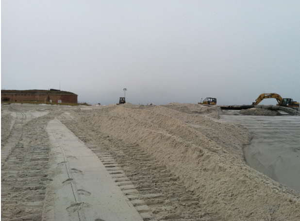
Over the 2011/12 winter, more than 500,000 cubic yards of sand were pumped on the north shore of West Ship Island.
