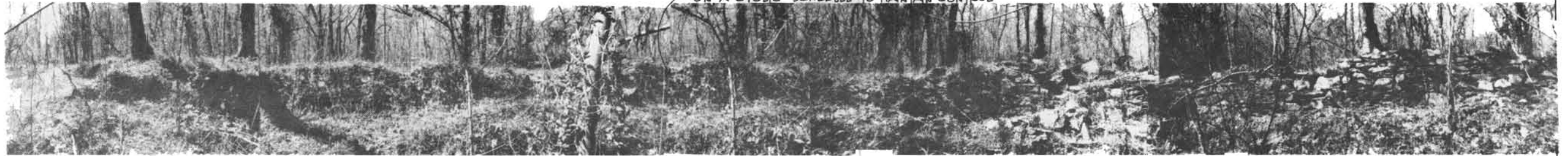
3 26 SOUTH END OF HOLDING BASIN WALL LOOKING WEST FROM OUTSIDE OF BASIN (PRIORITY 2F)
