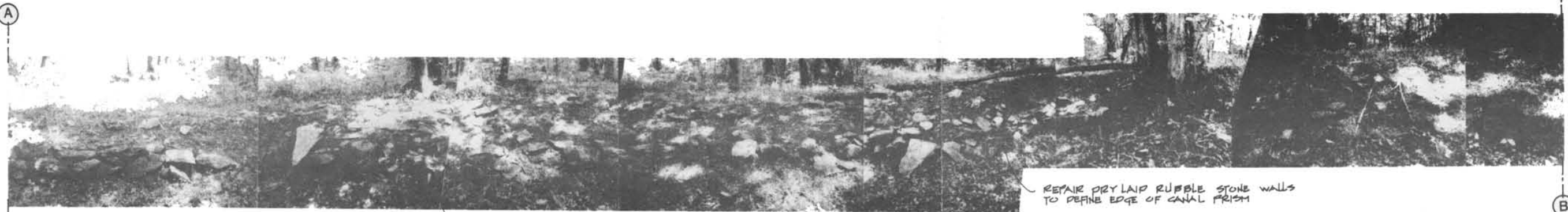
2 28 RIVER WALL - SOUTH OF HEAD GATE (PRIORITY 2E)
