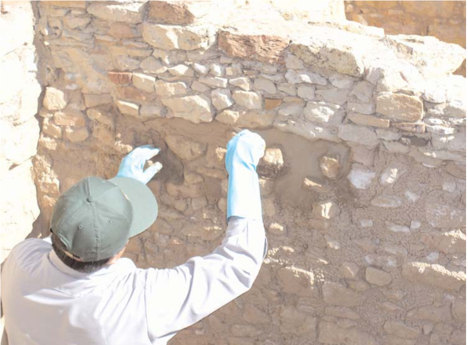
Figure 2. Vanishing Treasures masonry worker treating a void in a 700-year-old wall at Atsinna Pueblo, El Morro National Monument, New Mexico.
