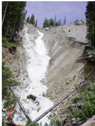
Figure 2. Grand Ditch Breach (Zone 1).
