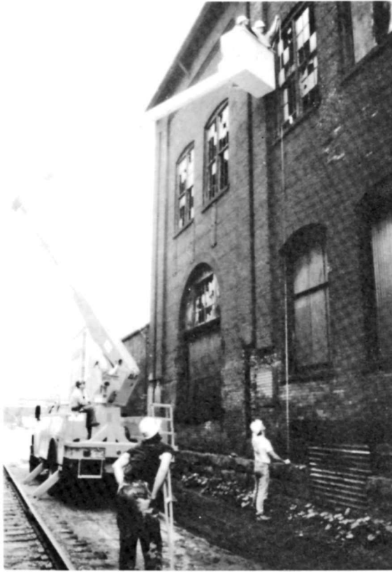
Dennis McGrath and Noel O'Dwyer ride a cherrypicker to measure the iron works building. Scott Clanton and Craig Strong assist from below. Photographer: K. Edward Lay, 1988
