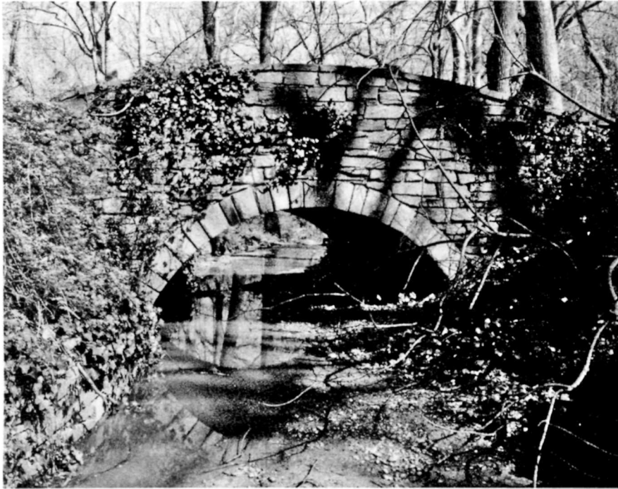
DUMBARTON OAKS PARK. Above , stone bridge. Below , using a plane table to survey the landscape are, l-r, Thomas Forde, Paul Dolinsky (project leader), Jacob Zemla and Andy Wenchel. Photographer: Jack E. Boucher
