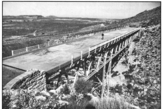
Dead Indian Canyon Bridge, Cameron vicinity, Coconino County, Arizona (HAER No. AZ-46). Photographer: Todd A. Croteau - 1994.
