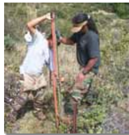
Park staff install and maintain fences to keep out destructive grazing animals.
